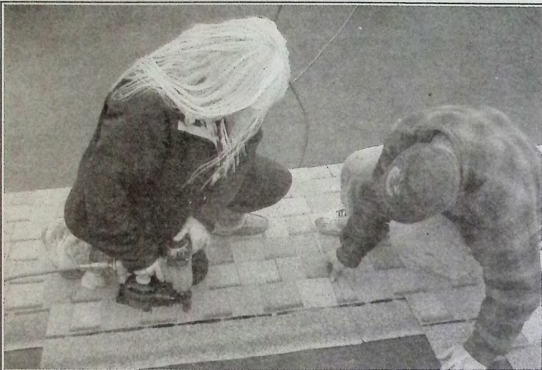
The News Leader's Brenda Engel shows the guys at All Purpose Roofing she's dangerous with a nail gun and gets the job done while helping shingle the Posse Training Centre November 6th.
