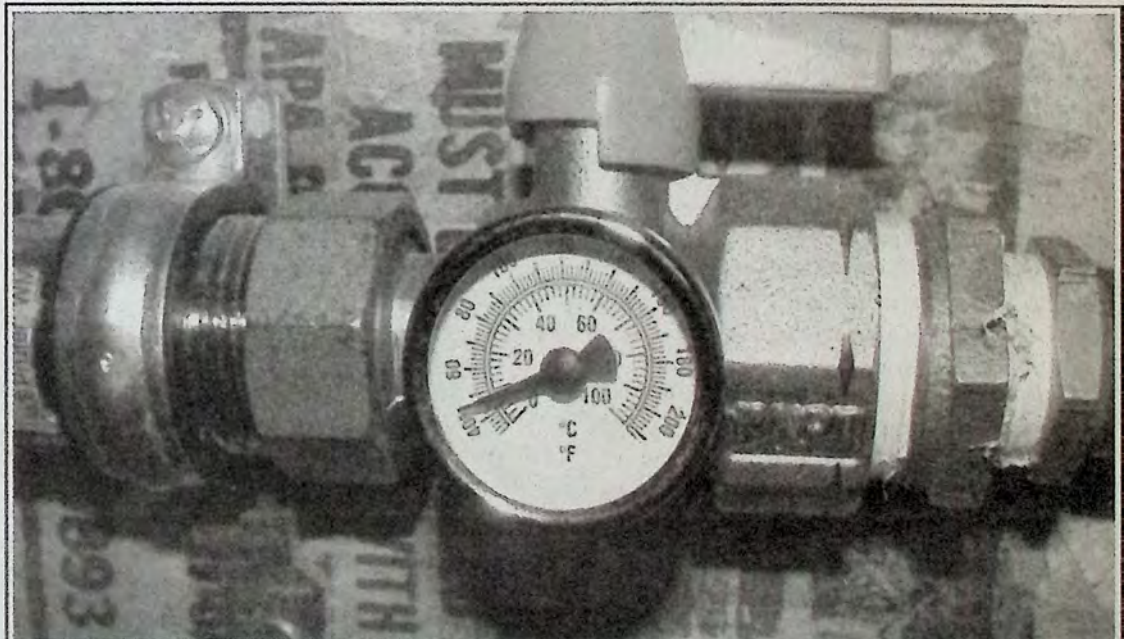
The cold water gauge shows a temperature of 47 degrees F. *
