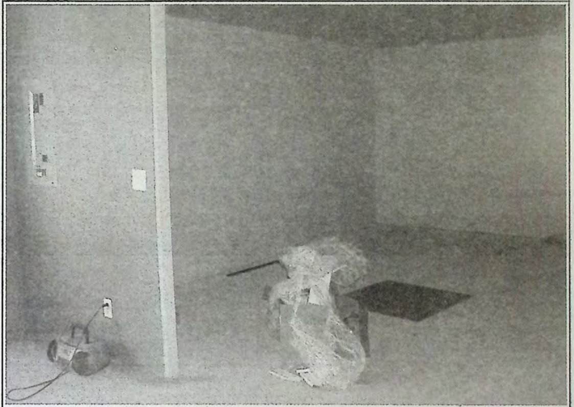
The Posse Training Centre continues to take shape. The walls were painted last week.
