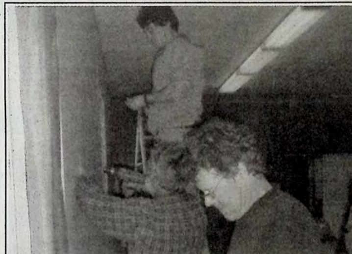
John Hutchinson ( foreground) Robert Mennell and Christopher Mennell (top) work on Cawston Hall renovation project.
