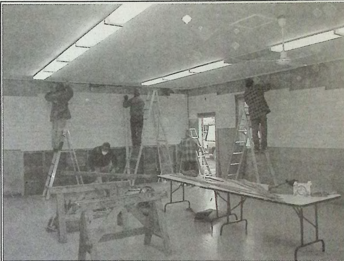
A look at work being done during the interior renovations. - photo submitted
