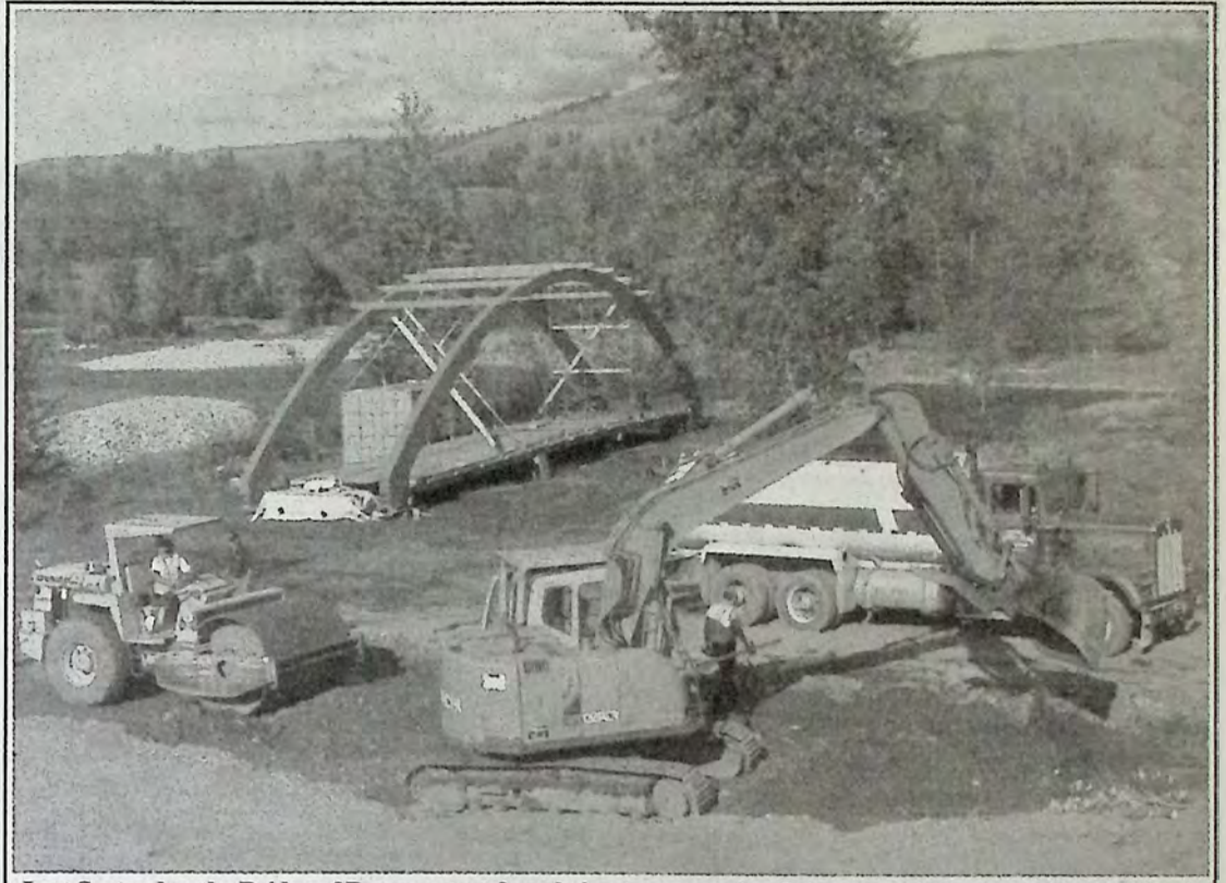
Last September the Bridge of Dreams went from being transported to Princeton to being assembled on site. *
