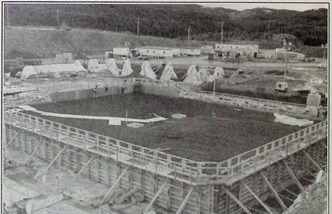
The SAG mill rebar and forms as the project looked weeks ago at Copper Mountain. - photo submitted
