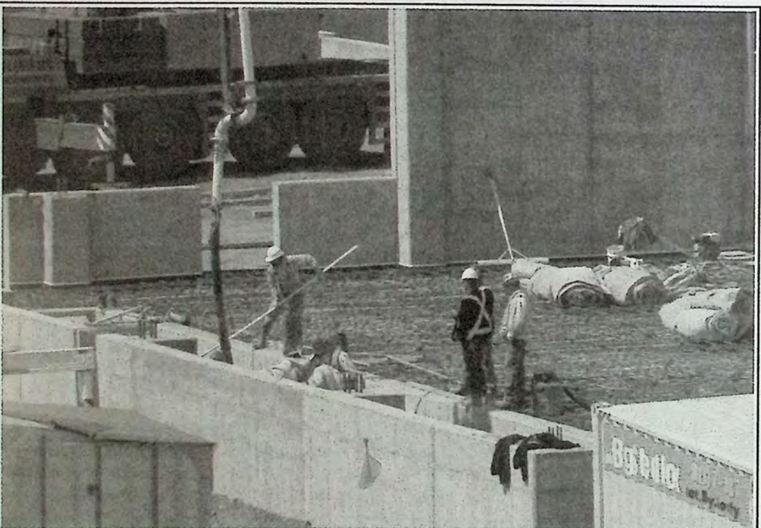
Concrete being poured at the concentrator building, Copper Mountain Mine May 8th. *
