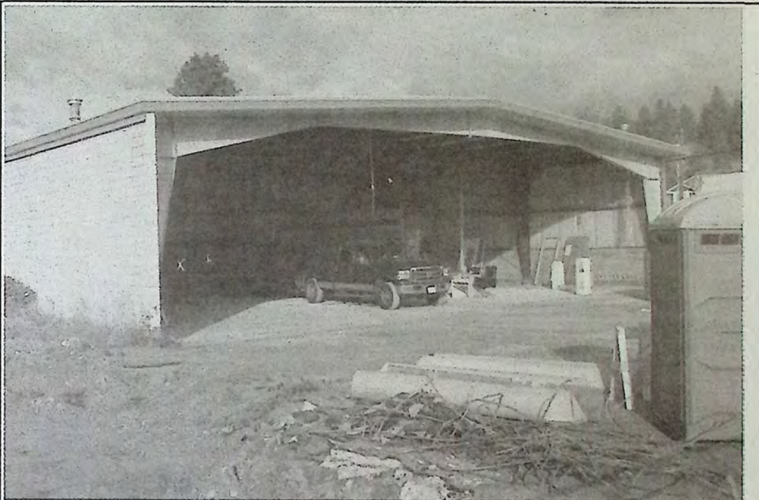
Last week the former Fields store on Bridge Street became a shell and a giant carport. Construction of the new grocery store will affect traffic downtown until October, according to the contractors. *
