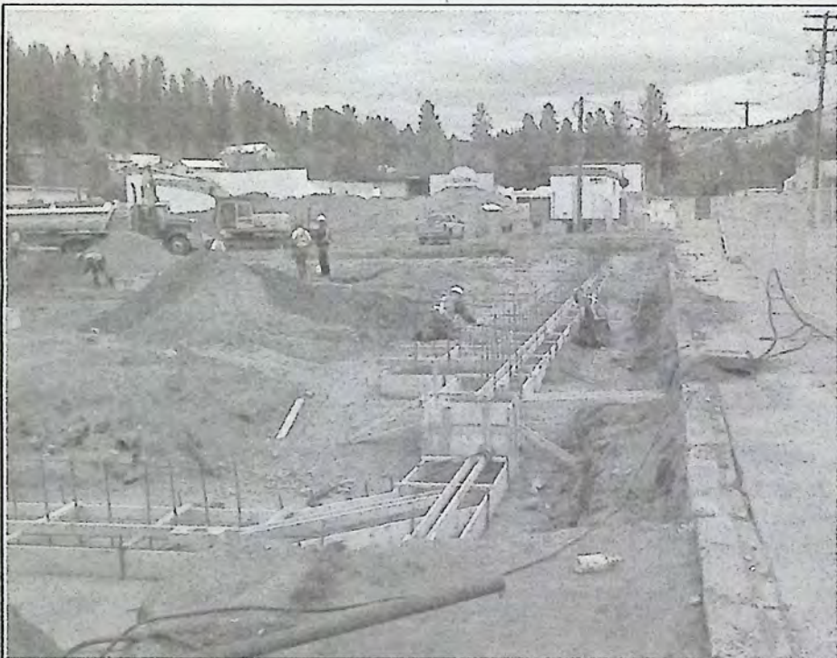
Another shot along Harold Avenue, this time looking towards Bridge Street. There is no parking allowed along Harold Avenue until October 31st. *
