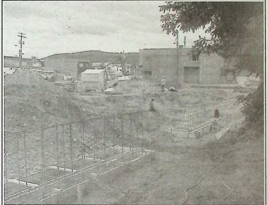
This shot from Angela Avenue looks across the back of the lot back towards Harold Avenue. The foundation forms give a sense of the size of the building. *
