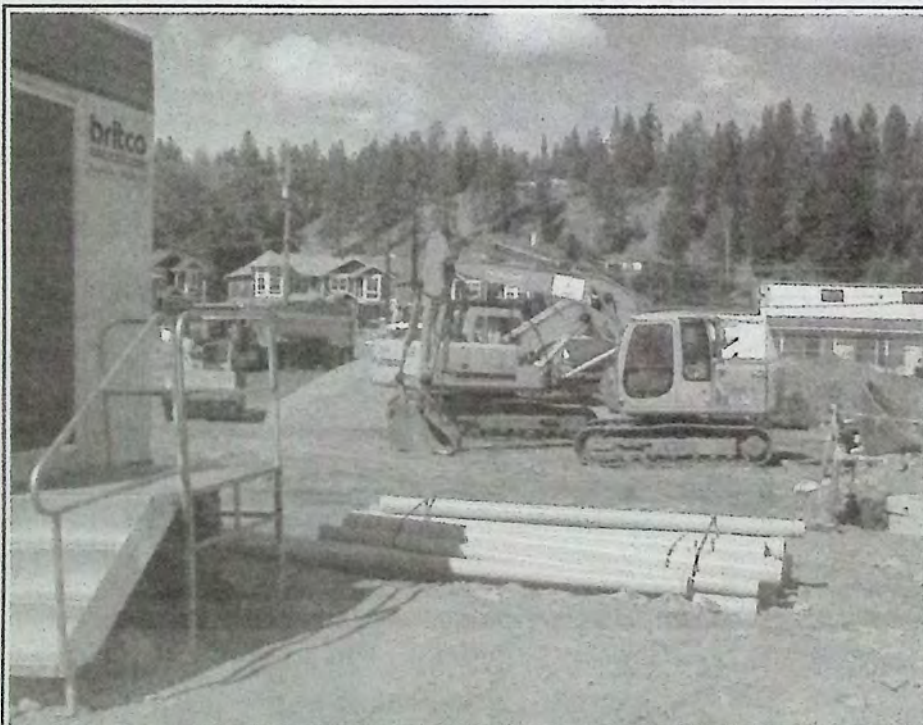
Angela Avenue has one way traffic, but no parking. One side of Bridge Street has no parking near the construction zone and the sidewalk is closed at the same location. *
