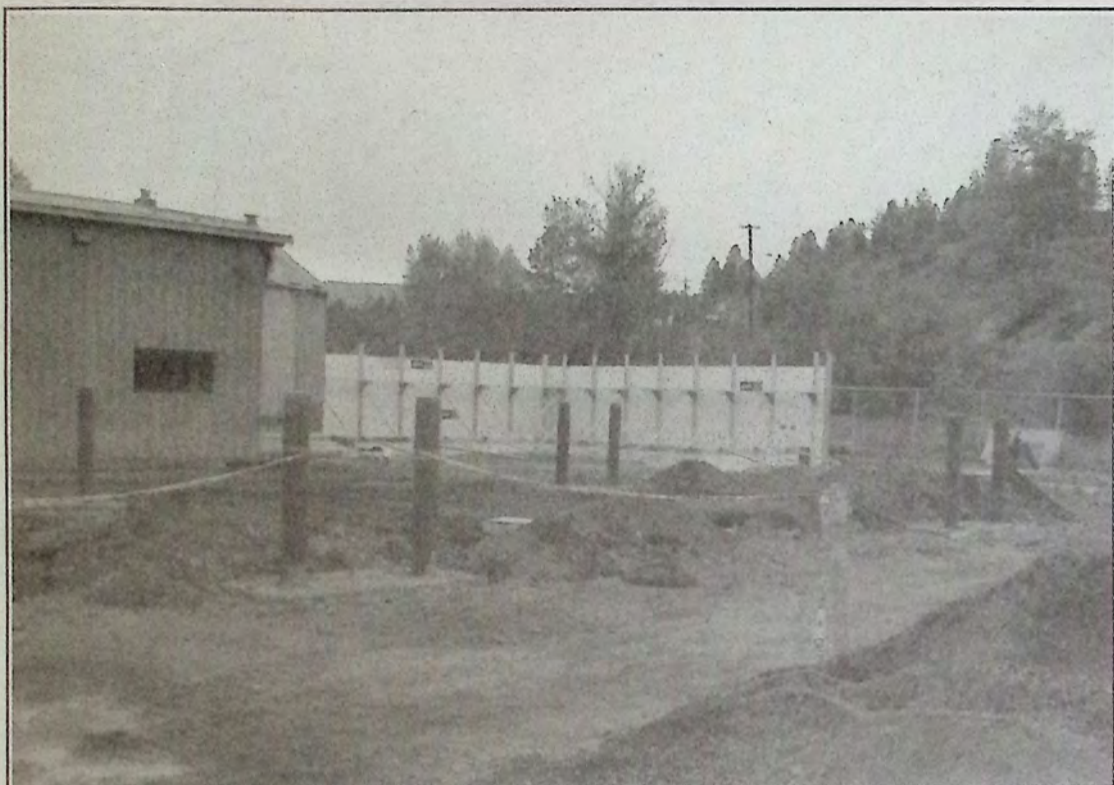
The commercial cardlock project on Burton Avenue has some residents in that area upset with the Town of Princeton feeling that the business should be in the industrial park rather than in a residential area. *
