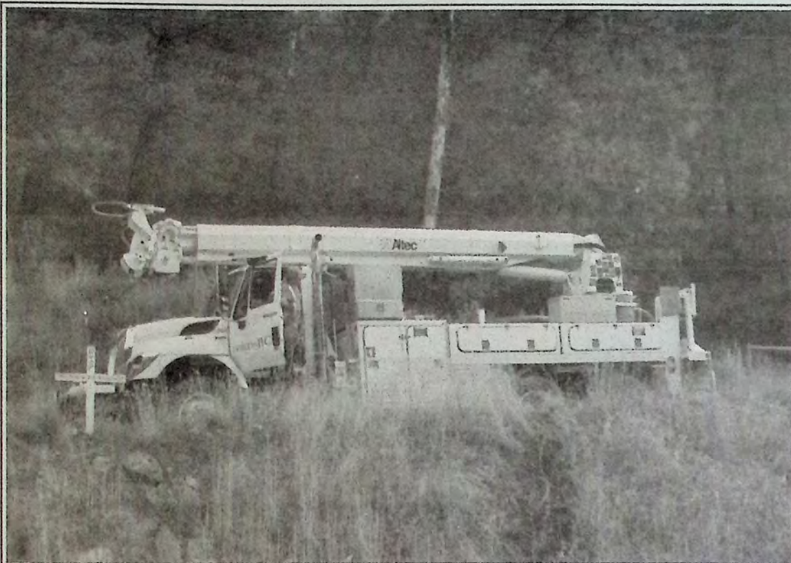
A FortisBC crew gets into position near Yellow Lake Saturday, September 25th. The Yellow Lake Safety Improvements Project is funded jointly by the federal and provincial governments as part of the federal Canada Action Plan to create jobs. The plan was launched January 27, 2009. The Yellow Lake project alone will receive $3,000,000 in federal funding. Photo: Arlene Arlow
