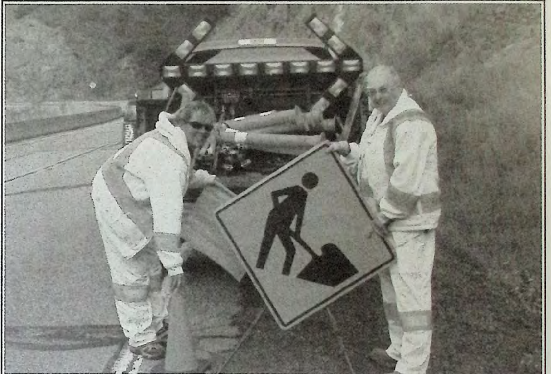
June Murray and Jeanette Clark of Central Interior Traffic Control were contacted at 6:00 PM on Friday, September 24th to perform flagging duties for Fortis BC workers the following morning as part of the Yellow Lake Safety Improvements Project. Photo: Arlene Arlow
