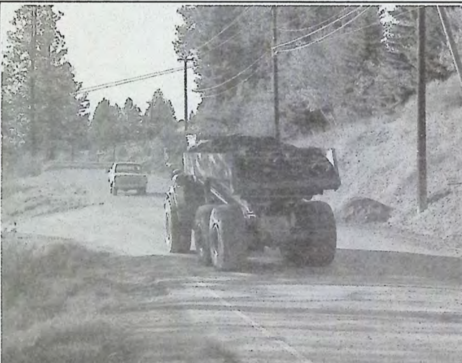
In addition to the water/sewer projects a total of seven paving projects were also scheduled for the month in various locations around town. Photo: Brenda Engel
