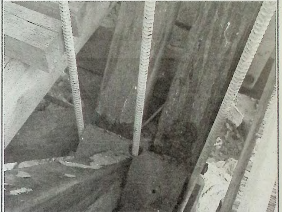
The view of three new metal rods used to stabilize the wooden bridge. The work on the structure has concentrated on replacement of a number of these rods. *
