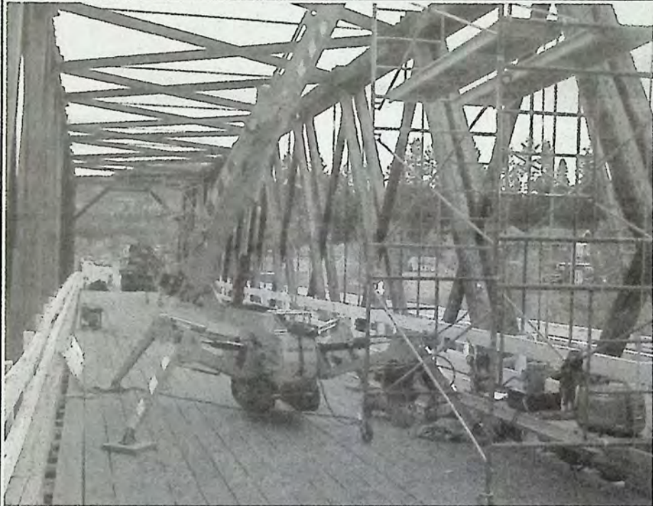
The wooden bridge at the end of Bridge Street has been closed to vehicle traffic since October 4th to allow for repairs to the structure which dates back to the 1930's. *
