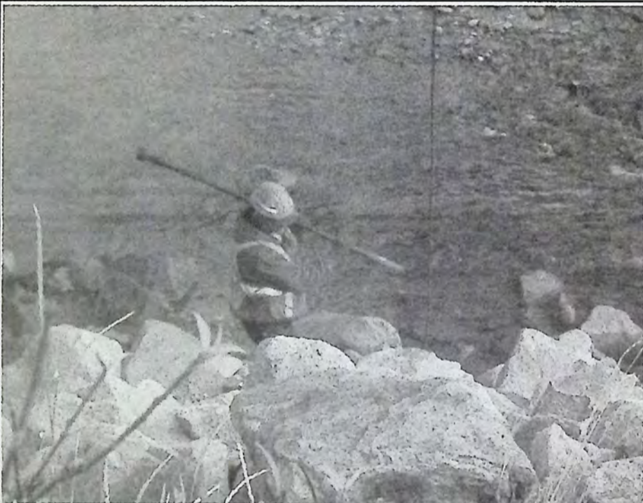
A member of the wooden bridge rehabilitation crew retrieves a portion of one metal rod that fell under the bridge once it was removed. A new one will take its place. *
