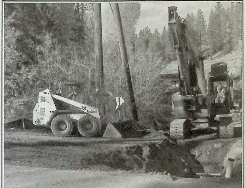
This was one of three water projects this month (Tulameen Avenue to Deerview, Bill Miner Way and Ingerbelle Drive) and a sewer project on Penryn Avenue. Photo: Brenda Engel
