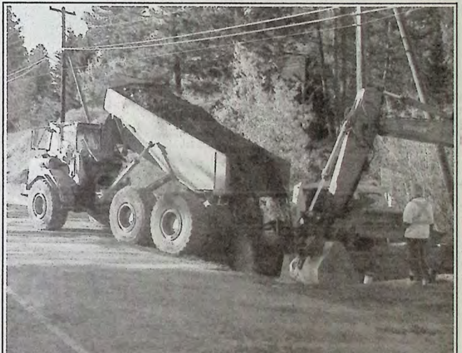
Crews were filling the holes required to join water main from Tulameen Avenue to service Ingerbelle Drive and Bill Miner Way residents on Friday, October 15. Photo: Brenda Engel
