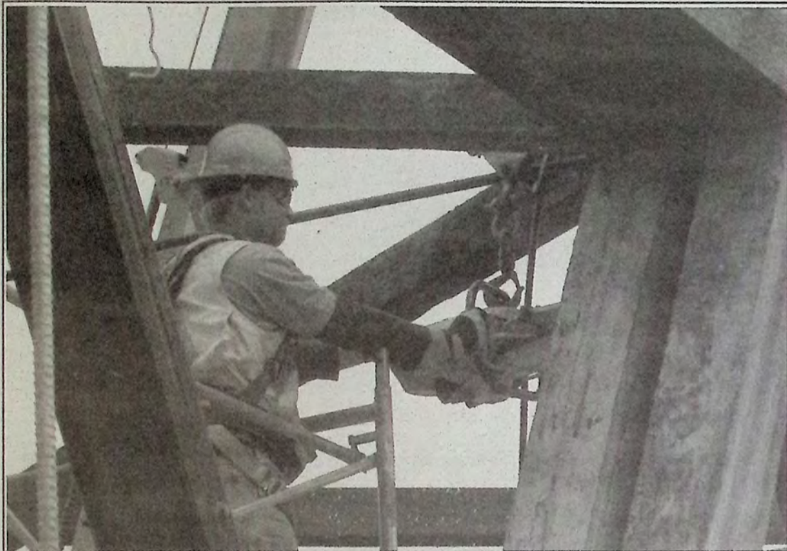
Crews are partway through the rehabilitation project on the wooden bridge at the end of Bridge Street which has closed the main route to all vehicle traffic. According to staff on site work is progressing well. *
