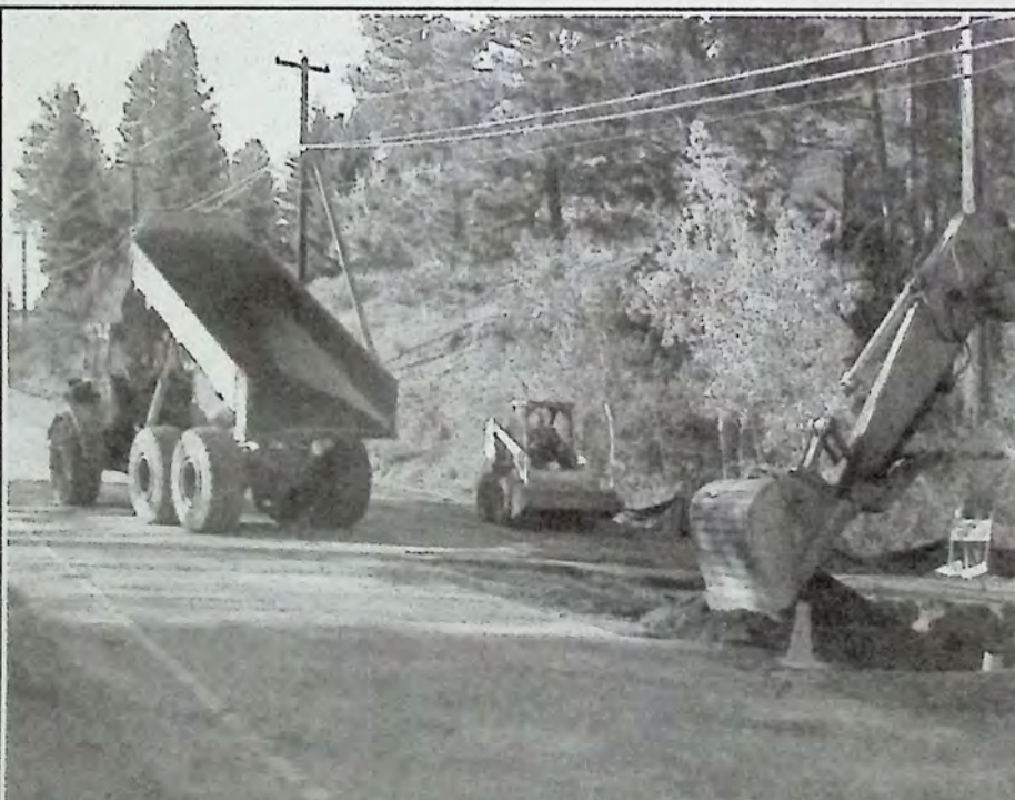
Residents are reminded to continue to expect minor delays in areas around Princeton as crews complete the projects. Photo: Brenda Engel
