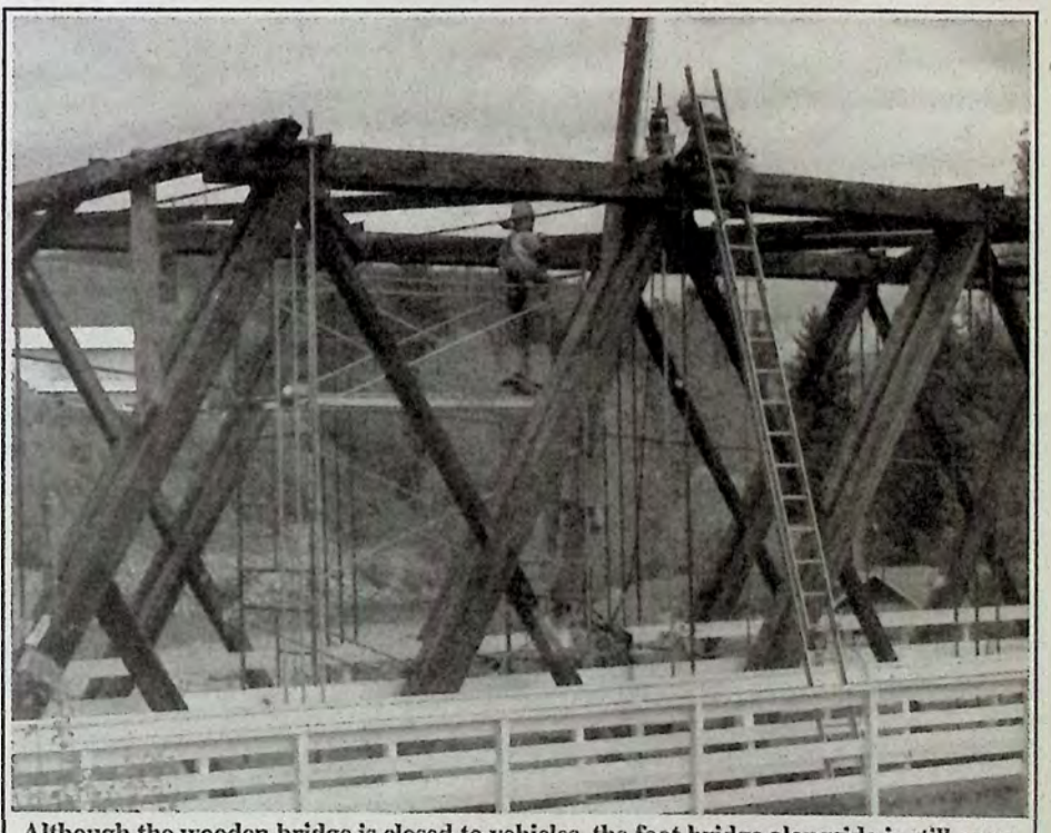
Although the wooden bridge is closed to vehicles, the foot bridge alongside is still open. This rehabilitation project is expected to be complete early next month. *
