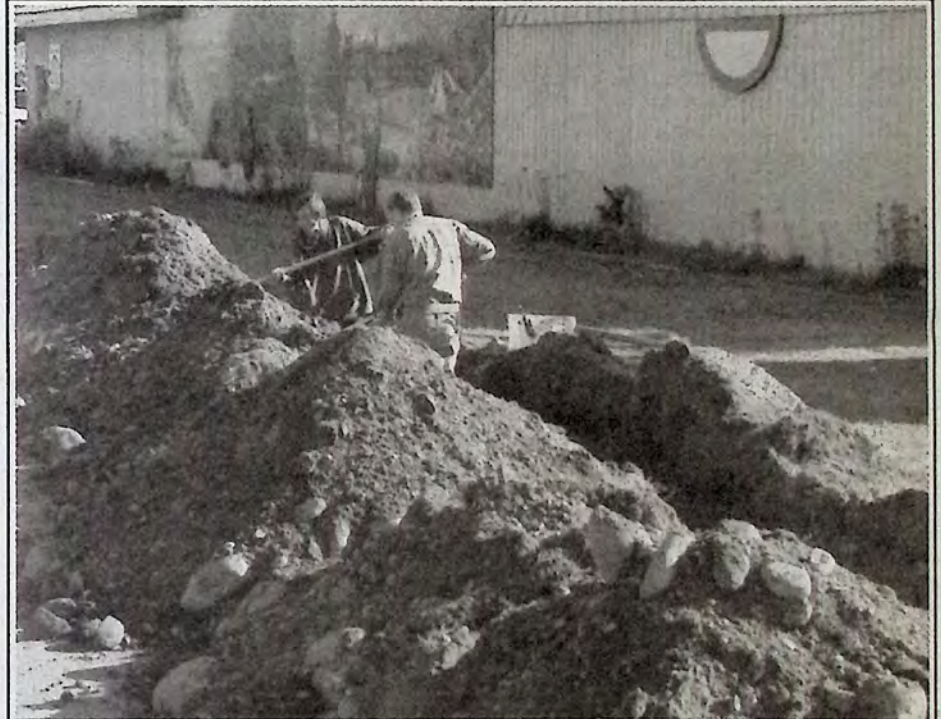
A look at a Hayes Creek Electric crew making sure all electric cables get laid properly and covered with a layer of dirt before back filling takes place. *
