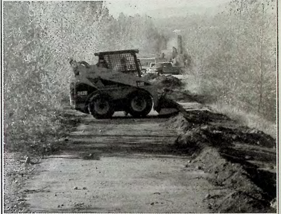
The finished project will see light standards along the trail from the Bridge of Dreams at the Tulameen River all the way to the entrance of the tunnel under Highway 3. *
