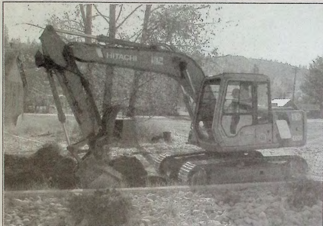
Stan Thompson of Model Transfer spent part of last week digging a trench to assist with the lighting project along the Trans-Canada Trail section that runs from the Bridge of Dreams to the KVR tunnel. *
