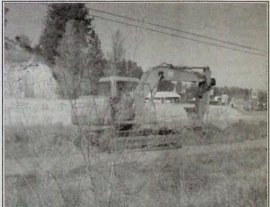
By lunchtime on October 21st Stan Thompson had made it to the back of the Princeton cardlock with the trench. The project will continue this week. *
