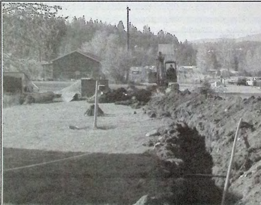
Another view looking west as Stan Thompson of Model Transfer gingerly digs the trench required along the Trans-Canada Trail along Burton Avenue. *
