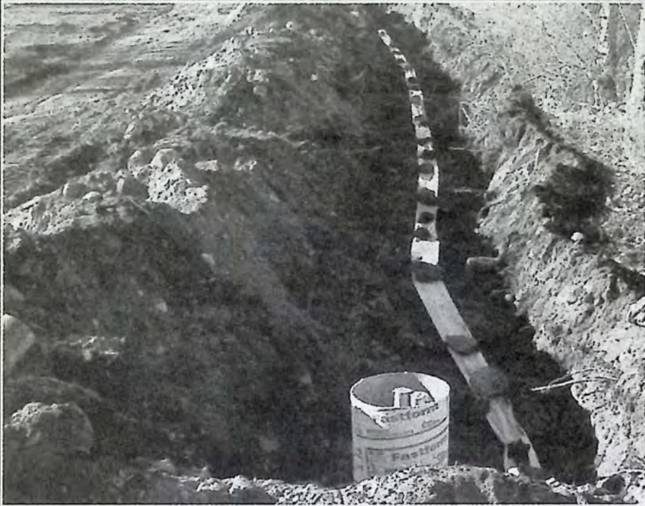
Work started last week on digging the trench for the underground wiring required in order to provide lights on the Trans-Canada Trail through Princeton. *
