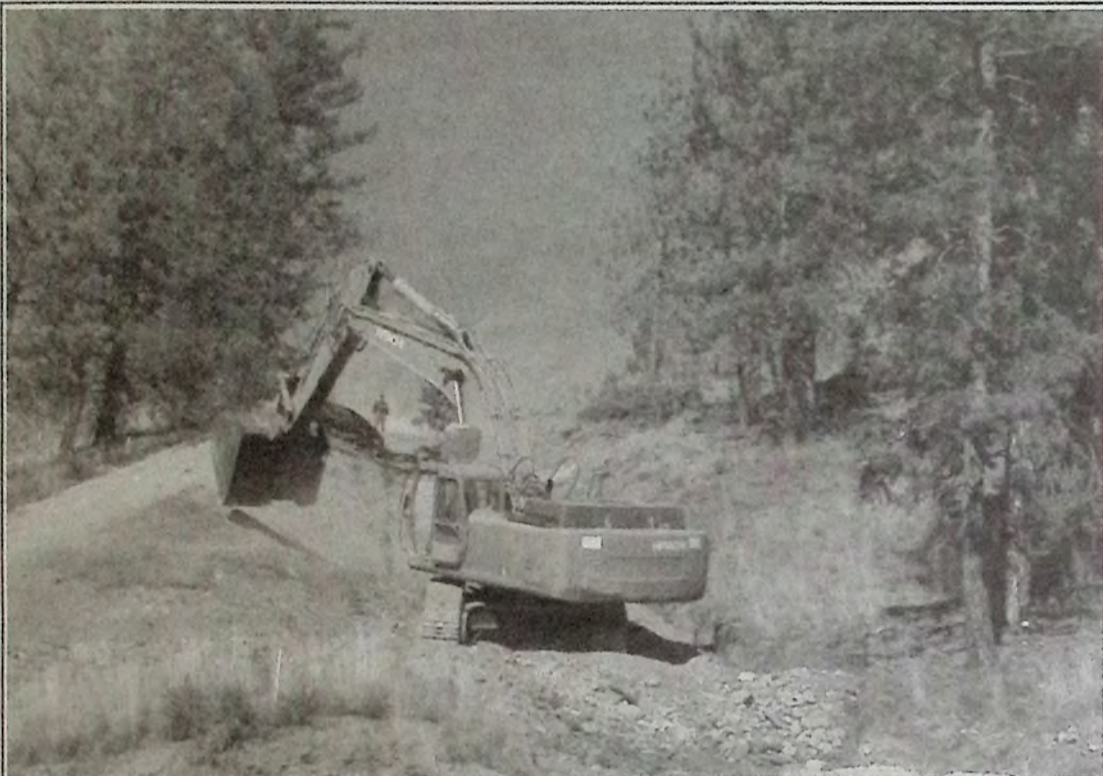
A crew worked last week on digging the trench for the new waterline which will run from the airport bench down to Bill Miner Way. It's one of many public works projects currently underway. Photo: Dawn Johnson
