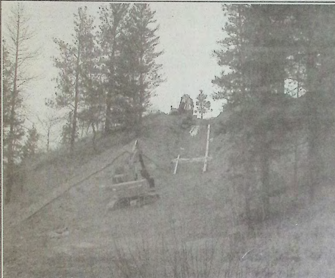
Last week, contractors worked quickly to complete the water line on the hill above Bill Miner Way. It has been a busy few weeks for the public works department in Princeton. Photo: Dawn Johnson
