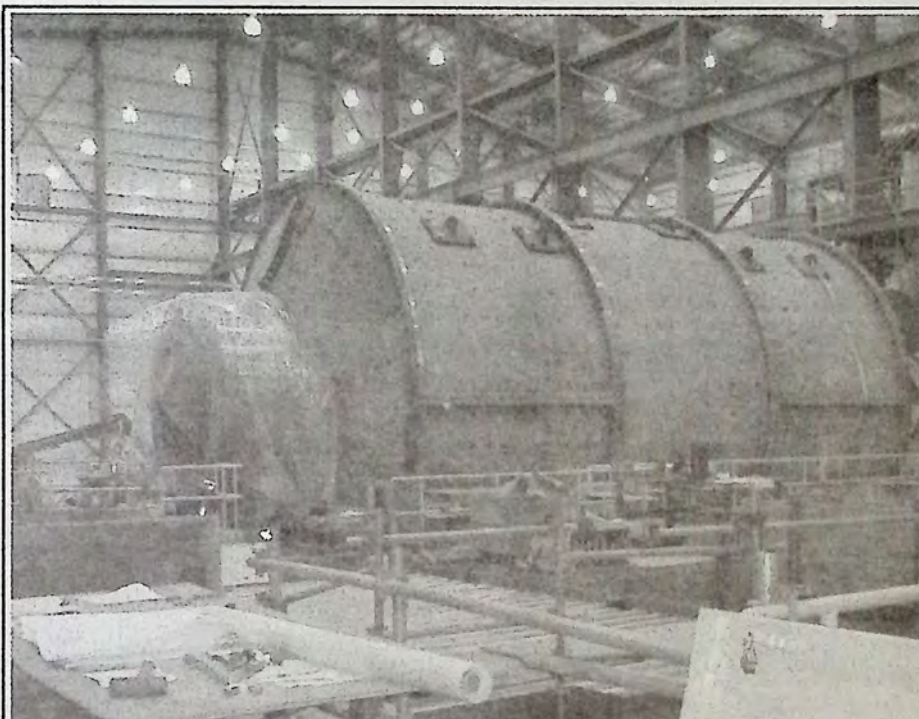
Part of the tour on November 18th at Copper Mountain Mine included a sneak peek inside the mill building, which is still under construction. *
