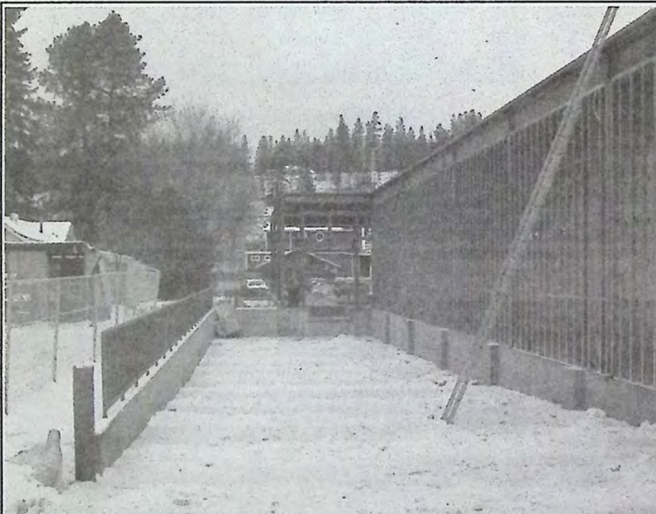
This is the view of the loading dock at the back of the new Cooper's Foods store. Food and supply deliveries will be left here with access off Harold Avenue. *
