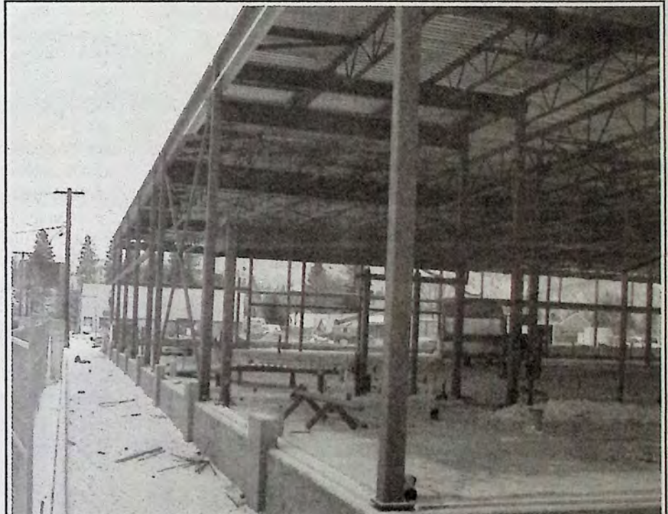
This is the view from the back corner of the building from Angela Avenue. If you look carefully enough you can see a portion of the existing Overwaitea Store. *
