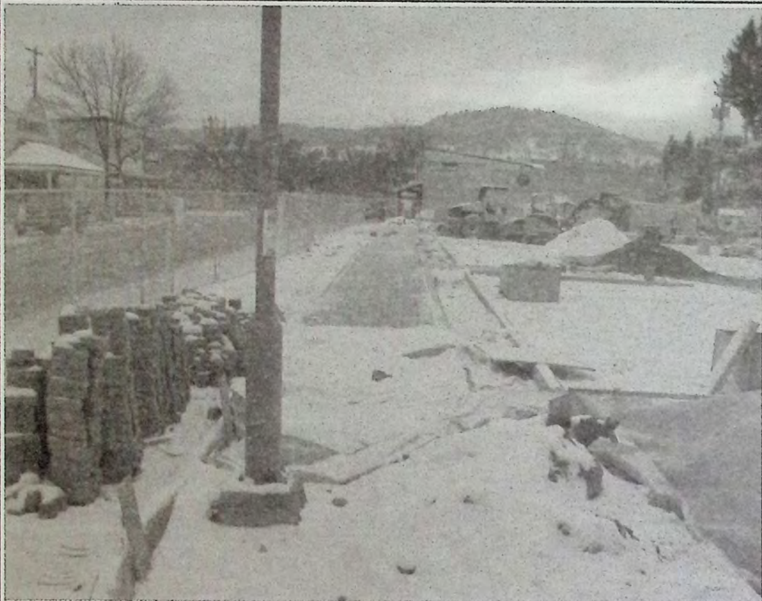
Although this section of sidewalk on Bridge Street in front of the new Cooper's Foods Store is closed for construction, it shows that there hasn't been very much snow in the area so far this season. A warming trend moved into the area late in the week and by Sunday afternoon some areas experienced melting. *
