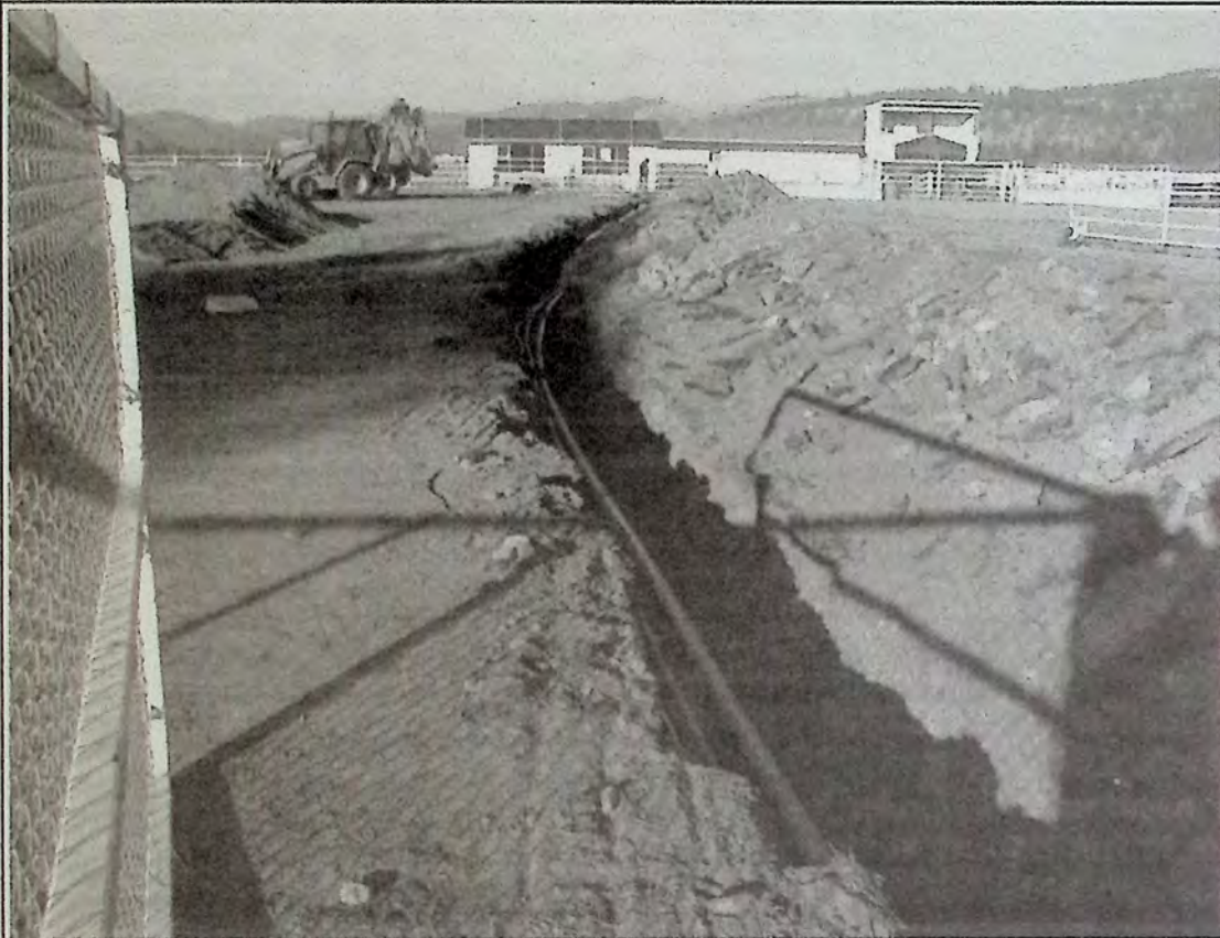
What looks like a bad case of gophers is actually work being done at Sunflower Downs November 28, 2008 to move services underground. This was the view across the race track and into the rodeo arena. *
