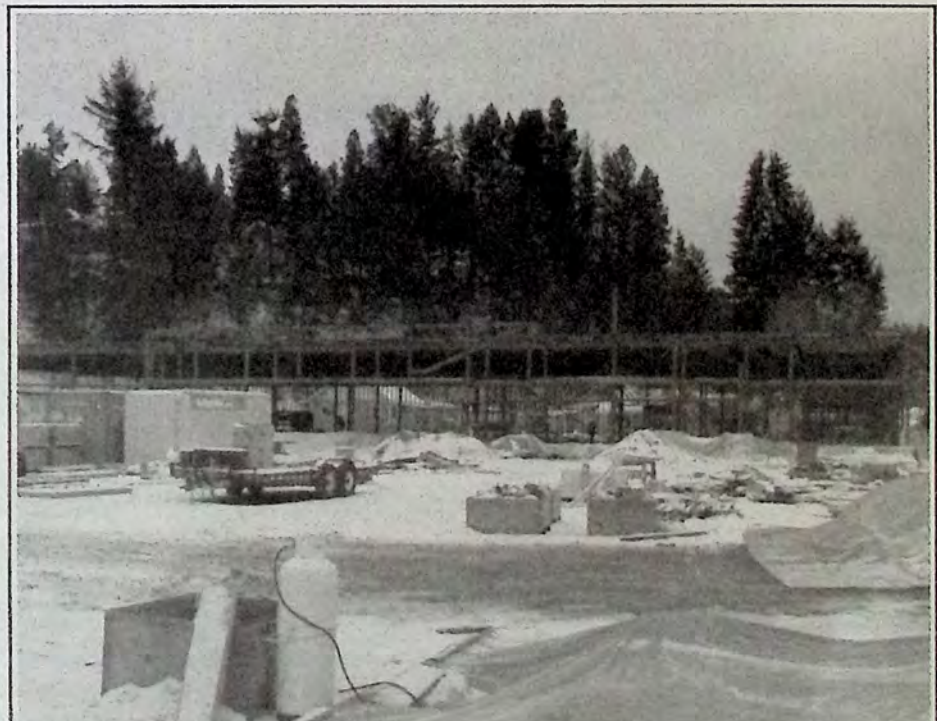
Looking from Bridge Street across the soon-to-be parking lot at the work being done on the new Cooper's Foods store in downtown Princeton. *
