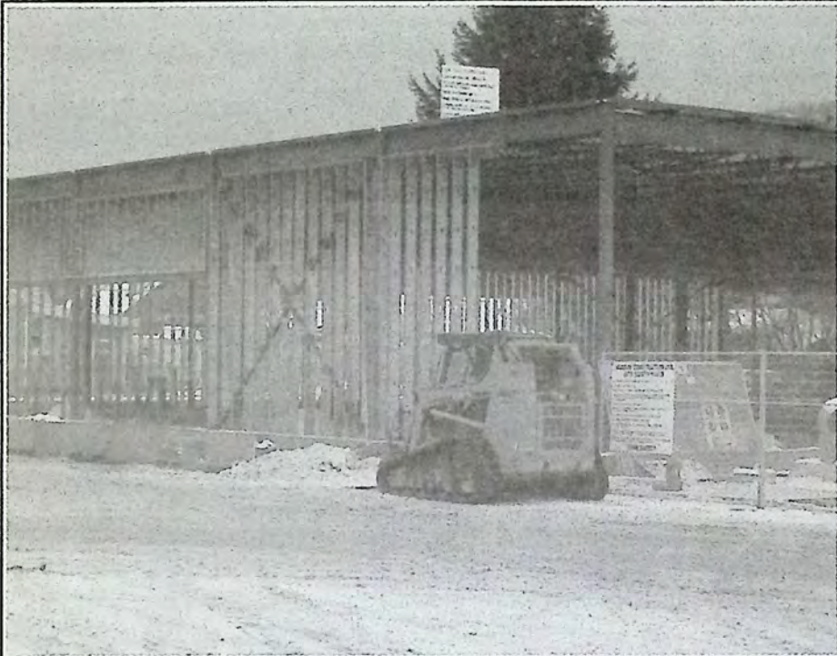
Progress continues to show on the new Cooper's Foods store downtown. This is the view of the front corner of the structure on Harold Avenue. *
