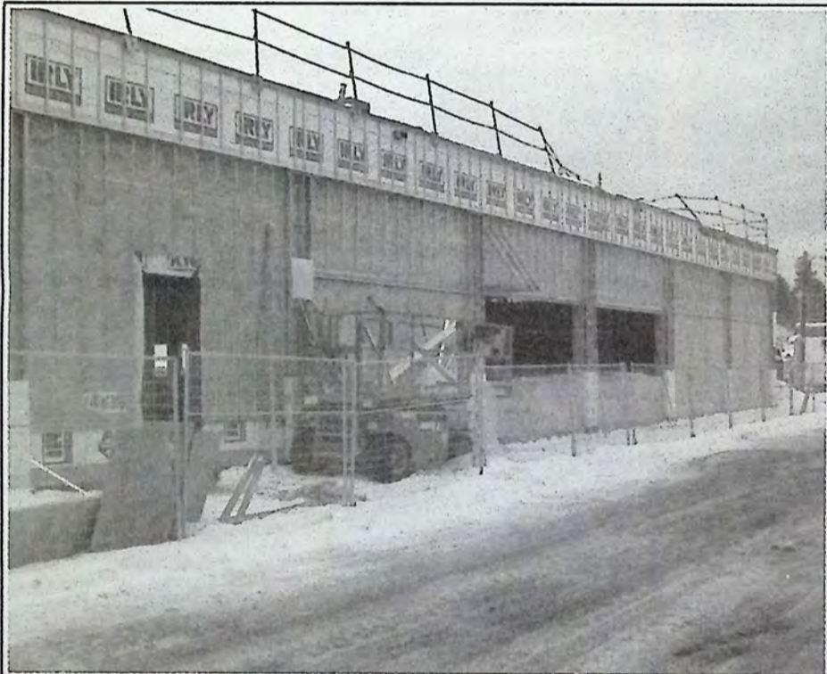
A side view of the Coopers Store from Harold Avenue towards Bridge Street. *
