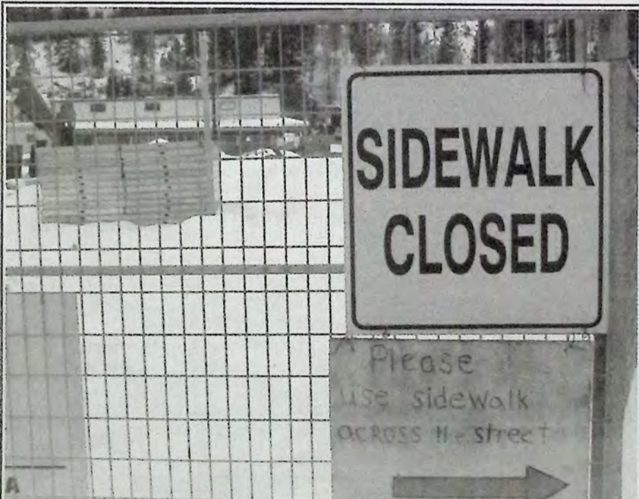
Progress continues to be made at the new Coopers Store downtown. This sidewalk, which runs along the front of the property on Bridge Street, remains closed. *
