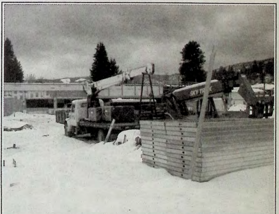
The front of the new Coopers Store looking from Bridge Street shows the size of the parking lot, which has been used for storage during the construction phase. *
