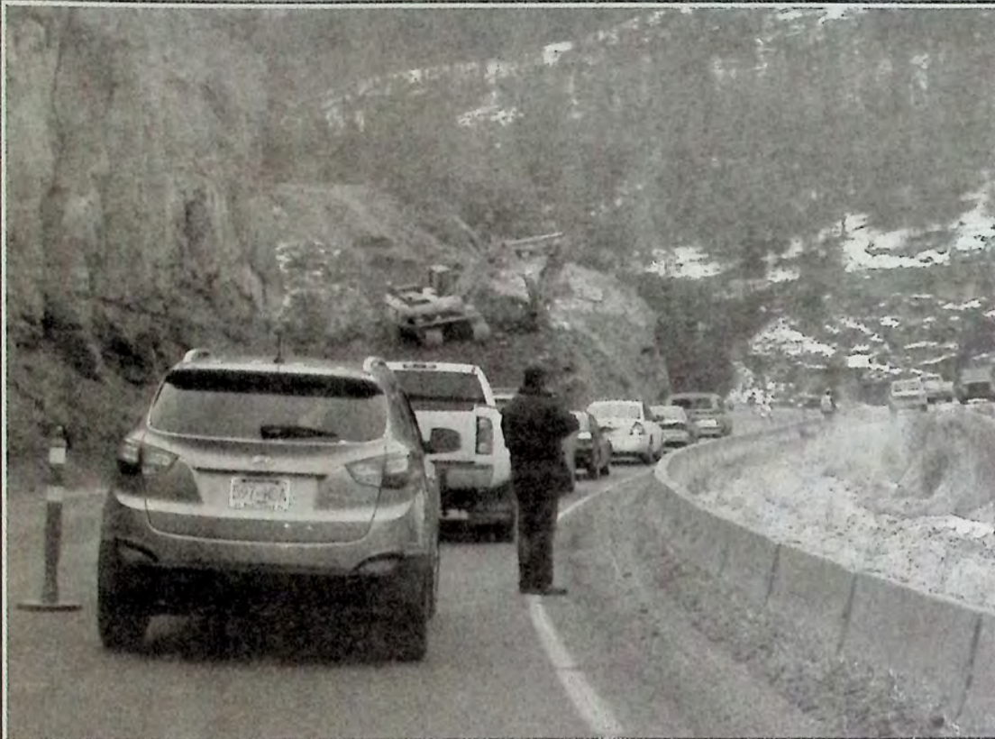
Construction at Yellow Lake is back on track after unforeseen delays. Stuart Cox of the Southern Interior Regional Office of BC's Transportation Ministry in Kamloops confirmed Friday, January 21st that blasting will start this week and continue well into the project. Traffic delays are minimal at this time but could be longer once blasting is underway. Photo: Arlene Arlow
