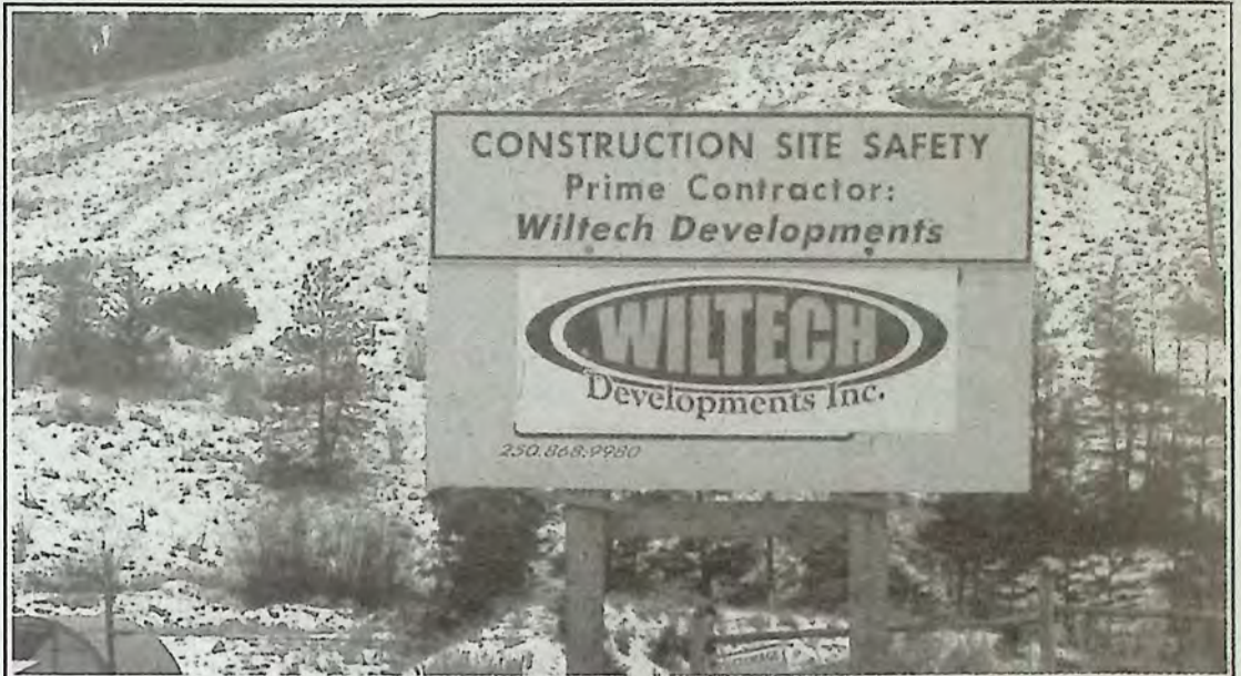
Wiltech Developments Inc. of Westbank has been signed as the General Contractor for the Yellow Lake road widening project. You will see their equipment and company logo onsite. Rampaul Dulay of the Interior Regional Office of BC's Transportation Ministry in Kamloops will take over as Project Manager in a couple of weeks. Rampaul confirmed Friday January 21st that timber from the site is being salvaged by Wiltech Developments. Photo: Arlene Arlow
