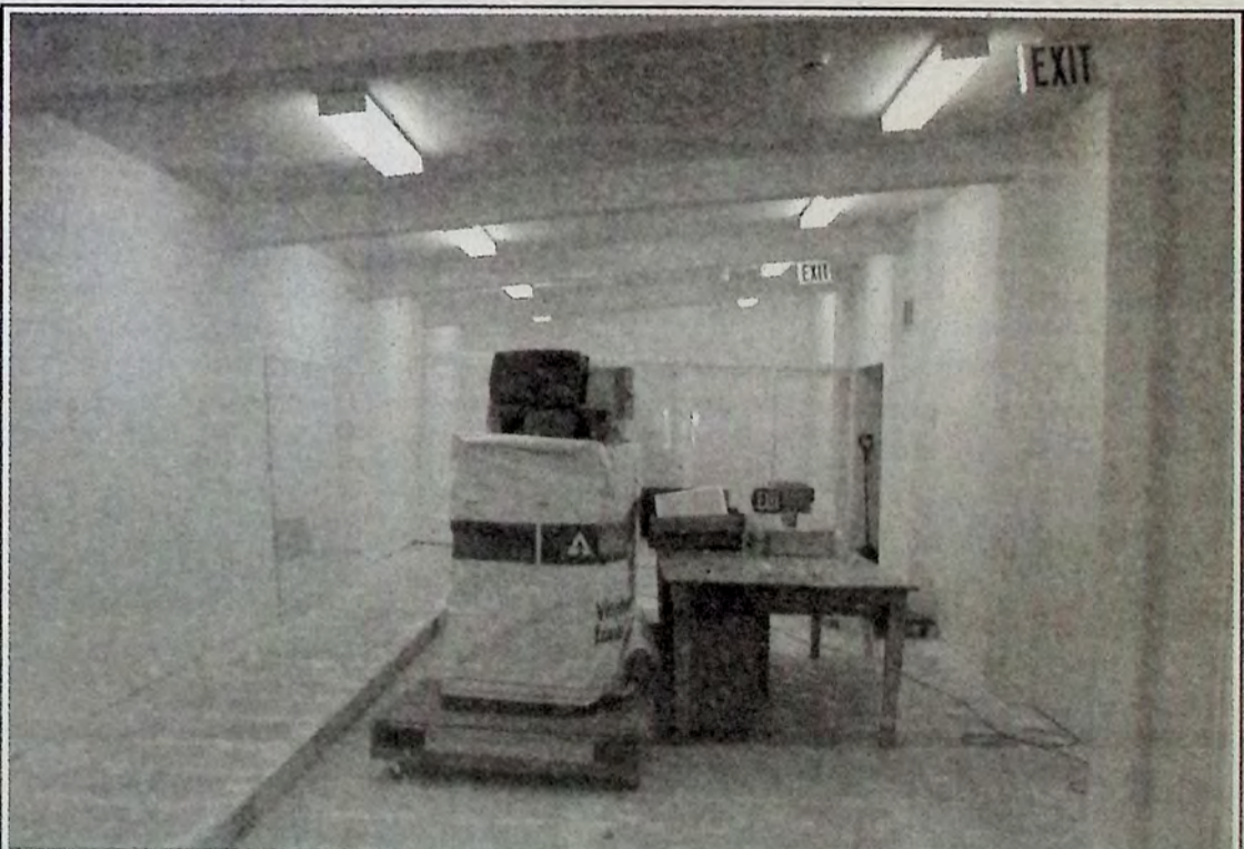
The Princeton Museum renovation project involves local contractors Fred & Company, Hayes Creek Electric and Ty French Heating. This is a look at the Pollard Wing last week. Photo: Terry Malanchuk
