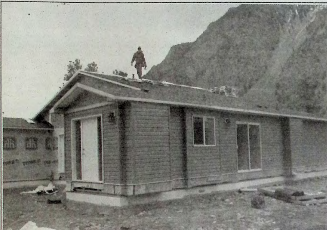
Justin Garner of Option One Exteriors in Kelowna performs roof clean-up duty for the Lower Similkameen Indian Reserve near Keremeos. A total of five homes are being built through joint funding with CEAP and CMHC. Photo: Arlene Arlow
