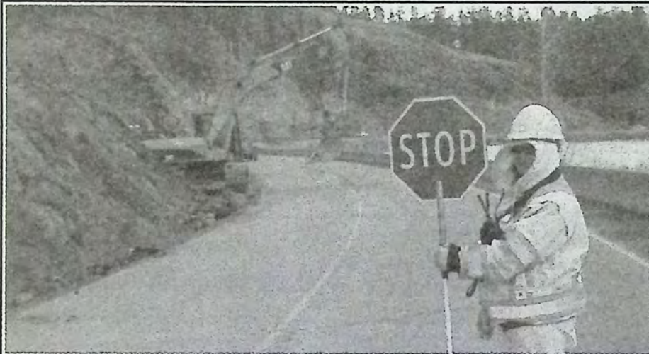
Tracey Borquest, TCP (Traffic Control Person) wears many hats - and many radios - for the Yellow Lake road project. Tracey is the Traffic Supervisor, keeping all the trucks and equipment as well as motorists moving safely around the site; she is the Site Safety Coordinator; plus she has First Aid Level III. She slings up to three radios around her neck at a time, listening to/communicating with the equipment operators and her counterpart Garry Lokstet (Traffic Control Person) who controls westbound traffic at the other end of the site. She takes her job seriously, but has had a few light moments, such as when a motorist tried to give her a 9-month old Siamese kitten recently. The motorist was trying to find the kitten a home. Photo: Arlene Arlow
