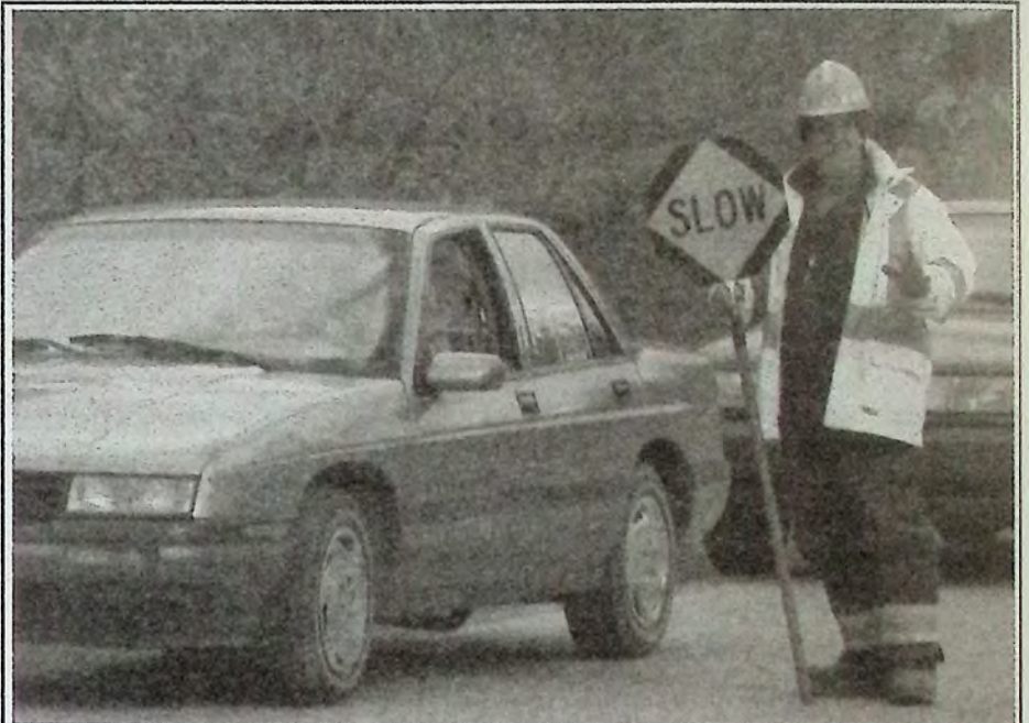
Garry Lokstet TCP (Traffic Control Person) controls westbound traffic through the Yellow Lake site. You will see a lot of Garry in the coming weeks: the project is anticipated to continue until late May. Give Garry a wave - he will always oblige with a wave and a smile if he isn't busy with traffic or on the radio. Photo: Arlene Arlow
