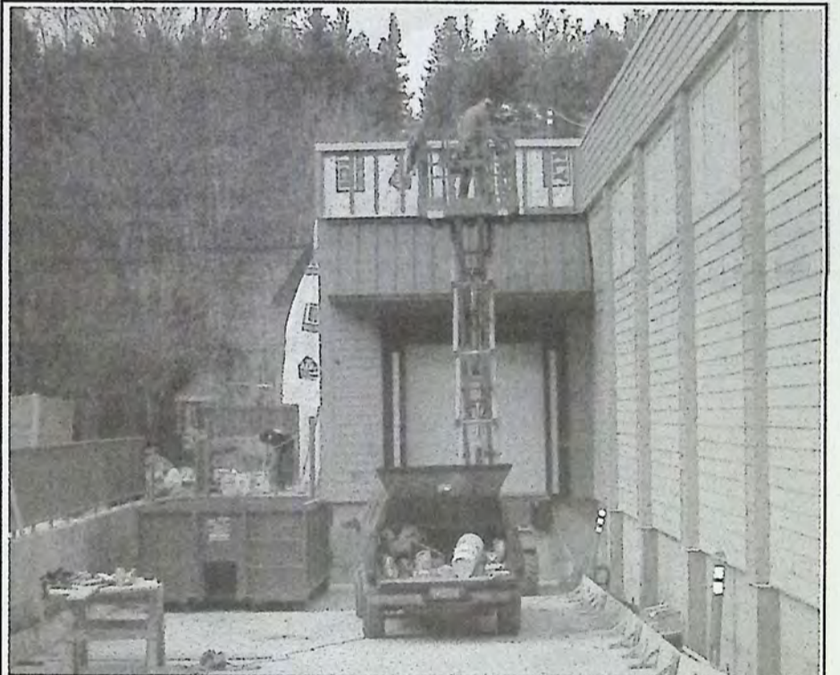
The rear loading bay looks finished with siding installed. Photo: Des Cosman
