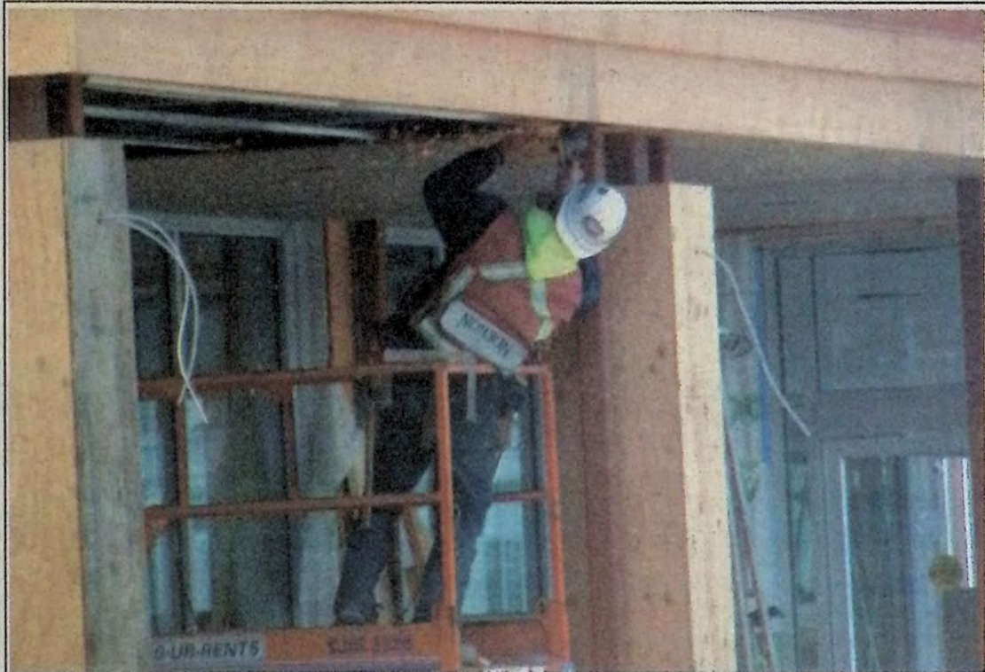
A member of the Norson Construction crew busy at work on the new Cooper's Store. Photo: Des Cosman
