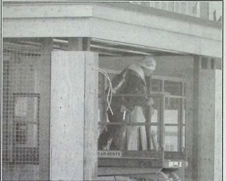
Norson Construction workers have been on the job for months. Photo: Des Cosman
