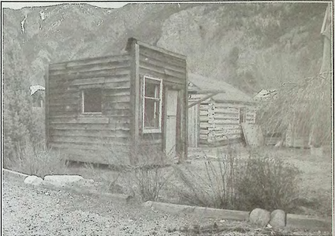
Building restoration work will continue on this former barber shop. Photo: Dawn Johnson
