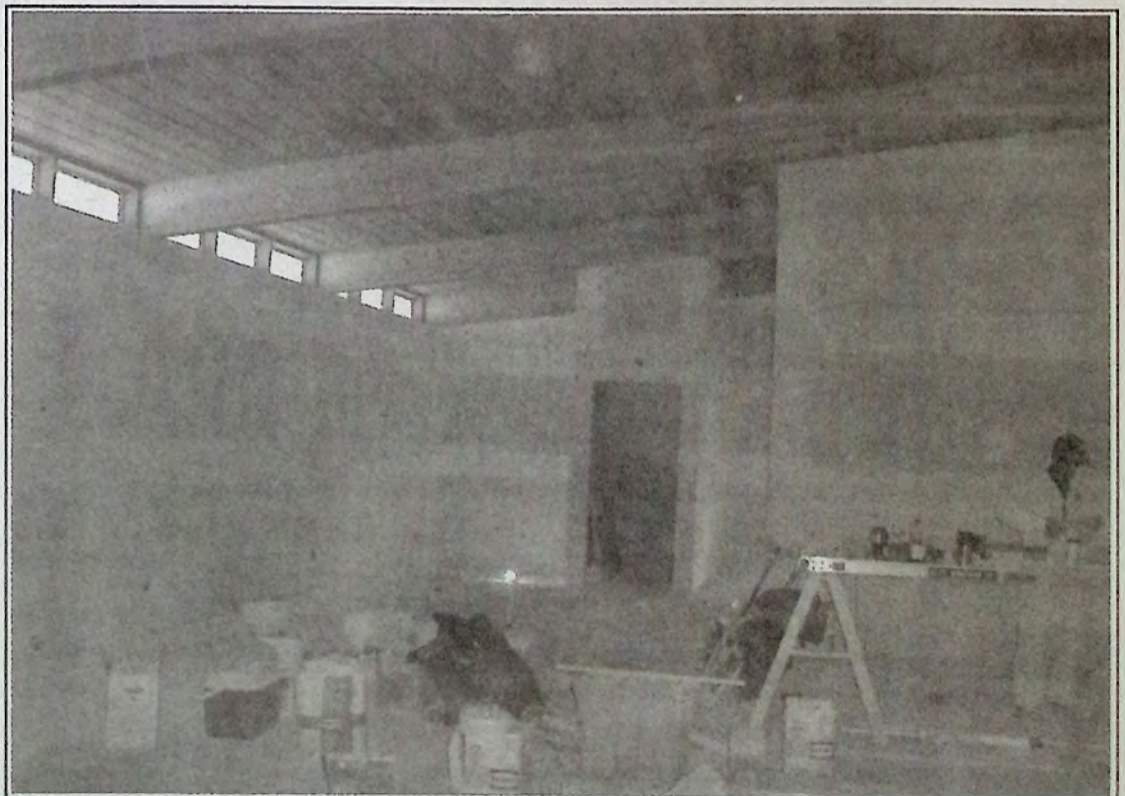
Another look at renovations currently underway at Princeton Museum. Photo: Terry Malanchuk
