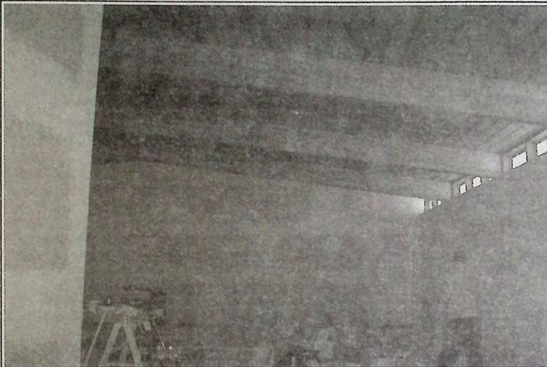
The former Library during renovations for the upcoming Museum expansion. Photo: Terry Malanchuk
