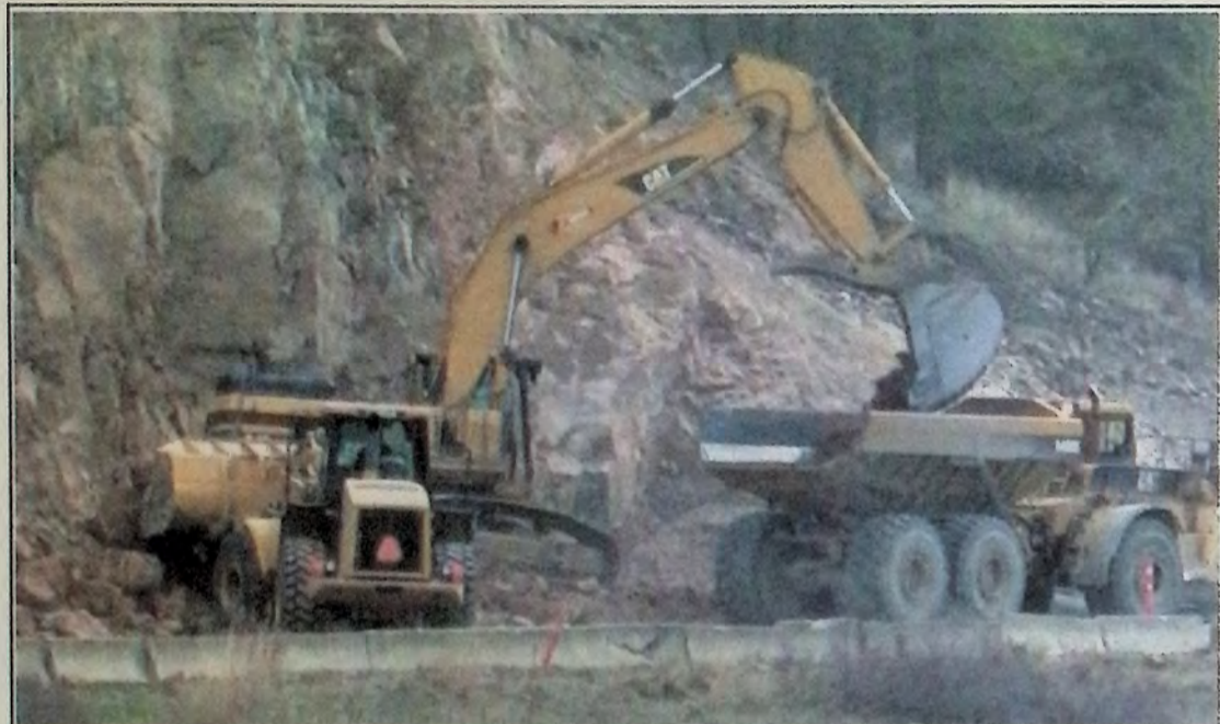
Following a rock blast, the loader operator piles up the rock and rubble while the hoe operator starts loading the heavy trucks. To witness the activities first-hand, you will want to arrive at the west end of the Yellow Lake Highway Improvement Project (eastbound) about four minutes after ten weekday mornings. You will experience a total delay of about an hour. More photos on Page 8. Photo: Arlene Arlow
