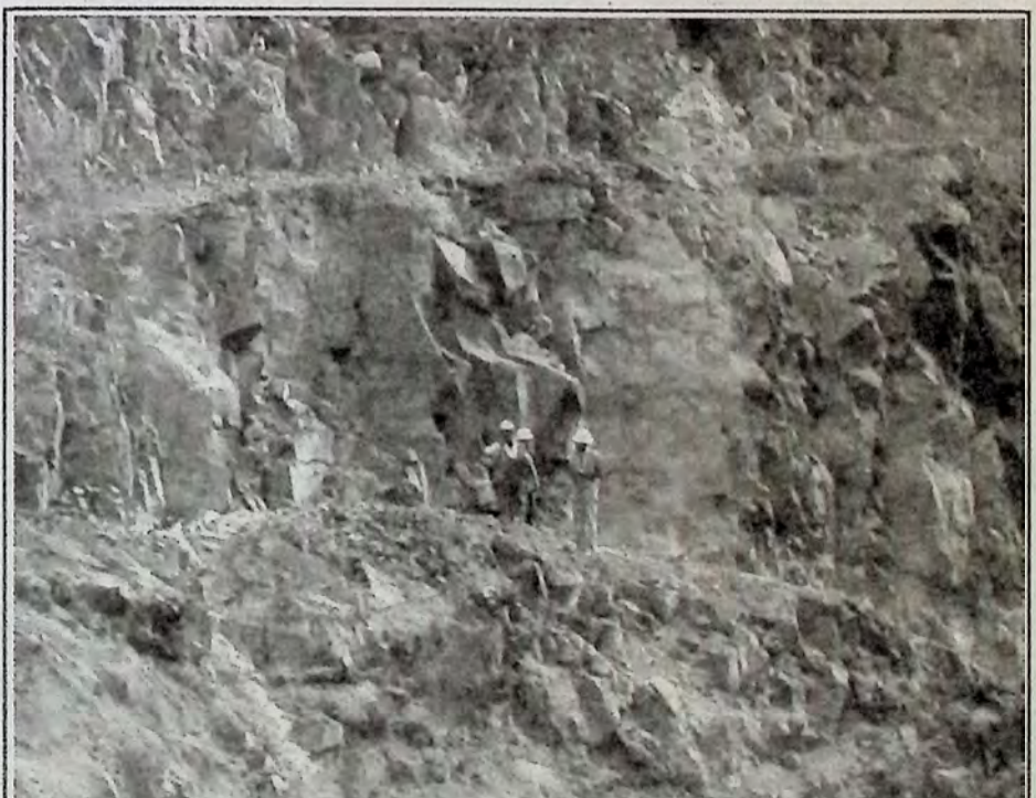
Site staff climb up onto the blast zone to analyze the success of the blast. The planning for the next blast and how much explosive will be needed starts all over again. Photo: Arlene Arlow
