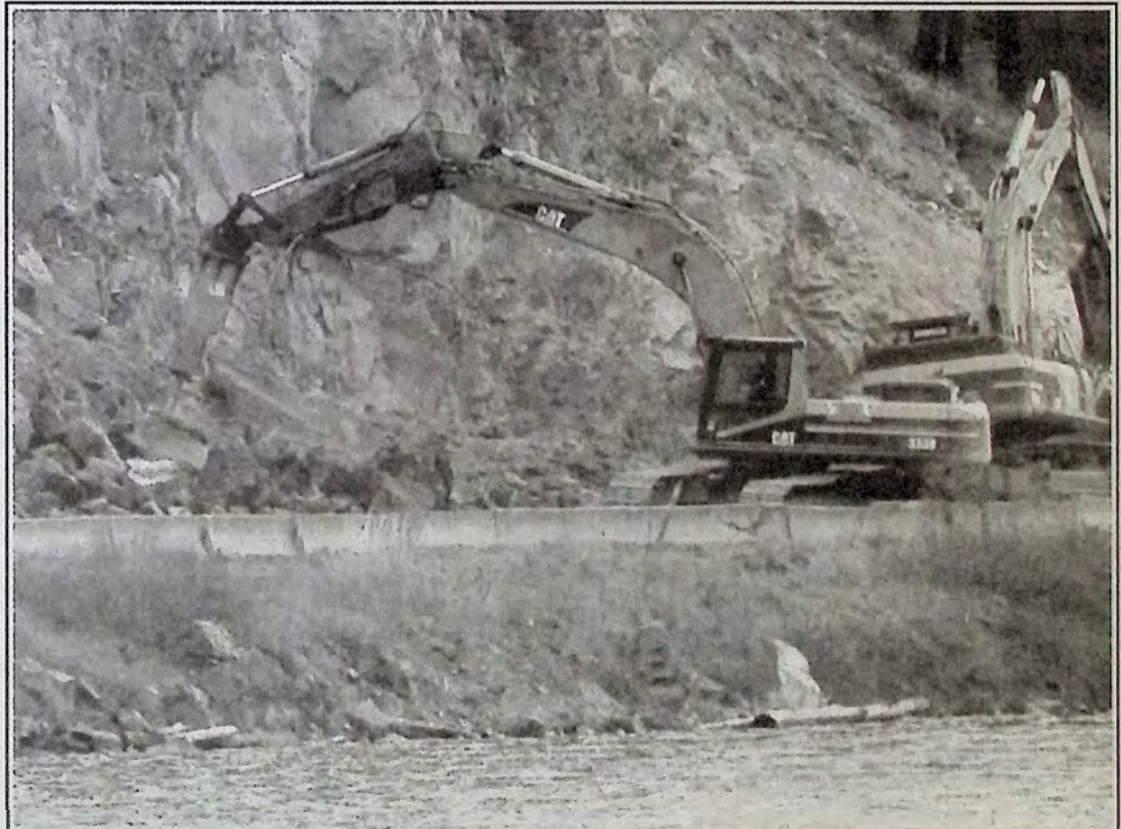
Following a rock blast at the Yellow Lake Highway Improvement Project, the hydraulic hammer breaks up the larger boulders while the hoe operator piles up the rubble for hauling. Follow the entire process from the beginning on Page 8. Photo: Arlene Arlow
