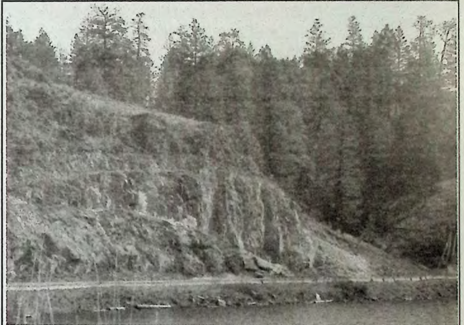
The explosive is set off. This photo was taken about a second after the explosive charge while the rock face was suspended in the air (up and to the left of the blast mats). Notice a couple of plumes of dust rising up within the rock face to the left and upward from the blast mats. Photo: Arlene Arlow
