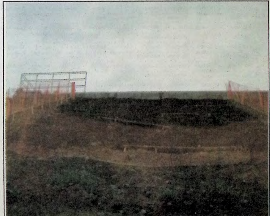
A look at the completed site surrounded by fencing. Photo: Morgan Dobbs
