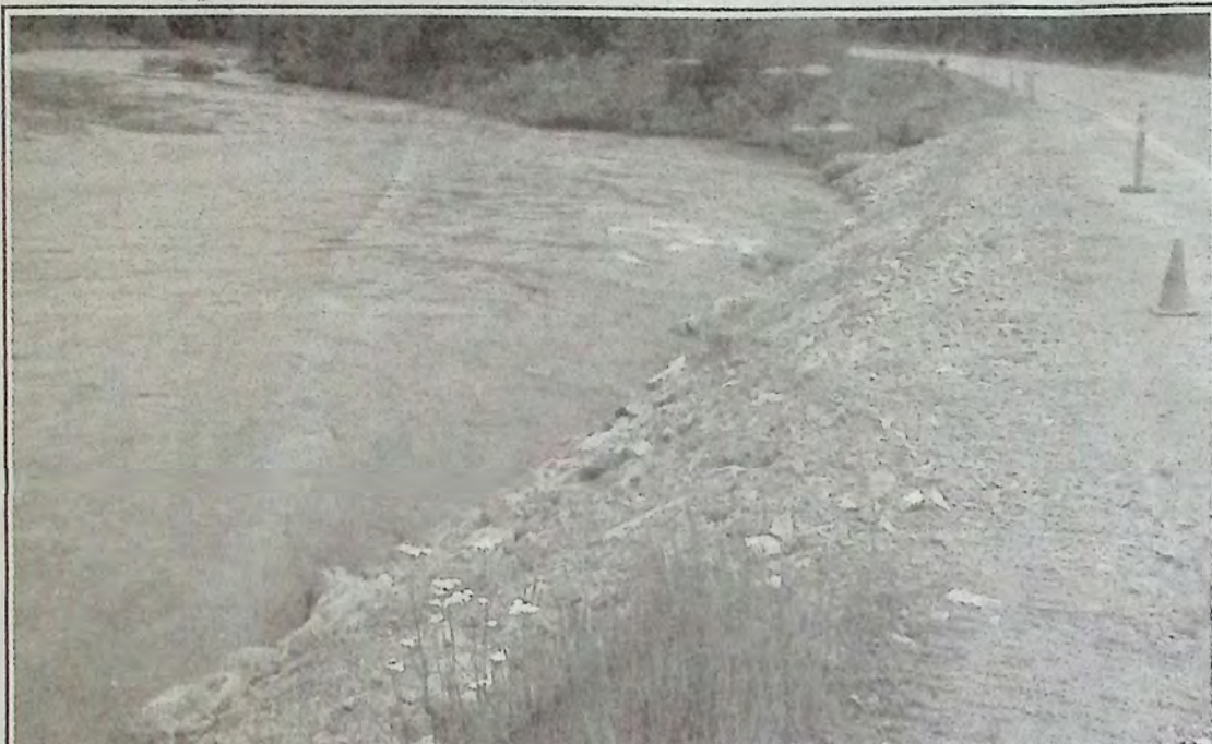
Highway 3 near Wolfe Creek received some extra material recently to keep Similkameen River from eroding away at it. The high water forced repairs of this nature throughout the valley. Photo: Brenda Engel
