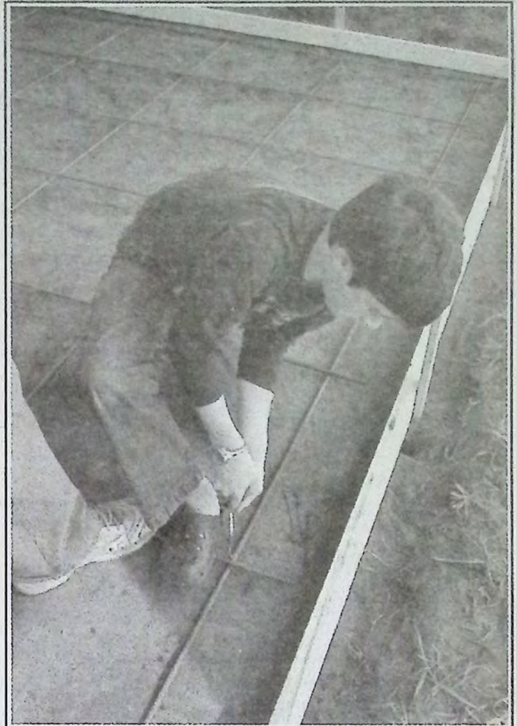
An important part of any concrete project is securing rebar. Princeton Secondary School students learned this and many more valuable skills as part of the YES2IT Program. Photo: John Kitts
