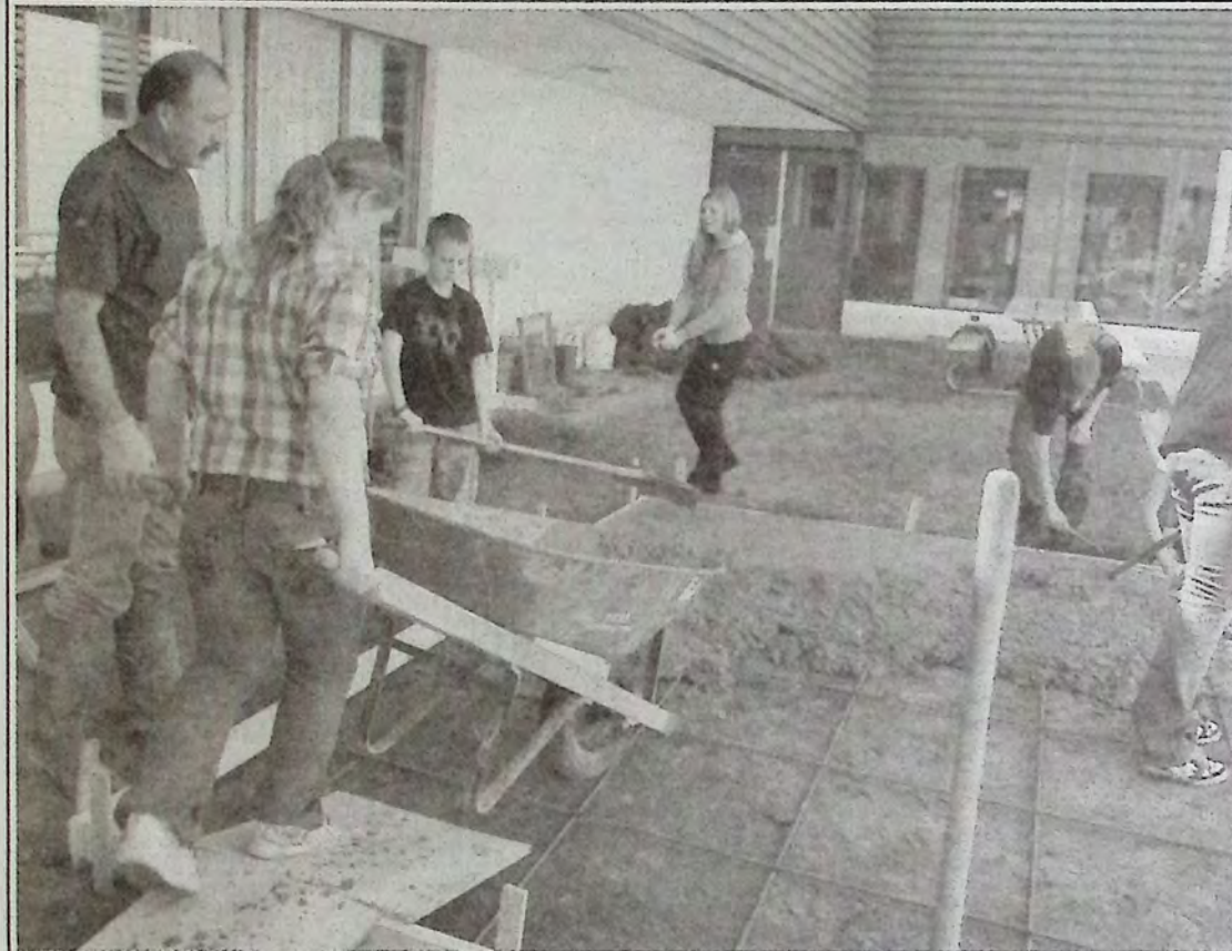
Transporting concrete to the job site involved a lot of work with wheelbarrows as part of the YES2IT Program at Princeton Secondary School. Students hauled concrete from the main entrance and across a hallway to the courtyard where a greenhouse was being built. Photo: John Kitts
