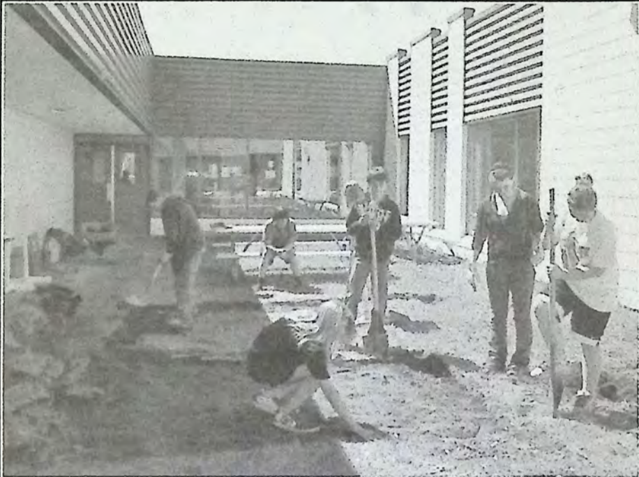
The YES2IT (Youth Exploring Skills to Industry Training) Program at Princeton Secondary School had students take a project from start to finish. Site preparation was the first order of business in the school court yard. Photos: John Kitts
