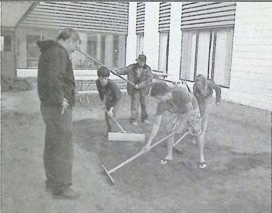
Once the site has been measured and grass removed, it is levelled which involves a lot of teamwork and organization. YES2IT teaches students these and other skills.
