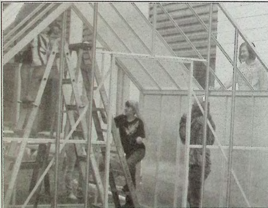
Students followed this project from site preparation to the finished product. Many local trades people were involved which added to the experience for students.
