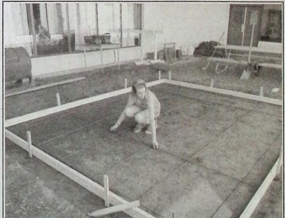
Rebar adds strength to any concrete project. Students learn the importance of this and YES2IT provides hands-on instruction so they gain a full understanding.
