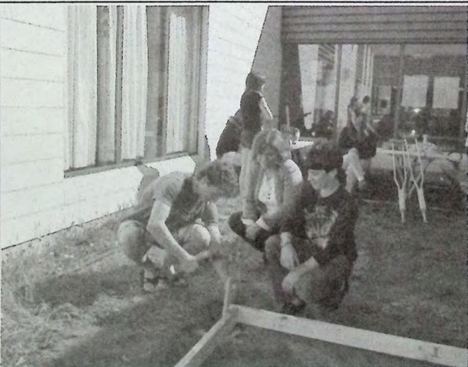
Before concrete can be poured to make a foundation pad, forms need to be cut and installed. Students show Principal Sandee Blair how to secure the foundation frame.
