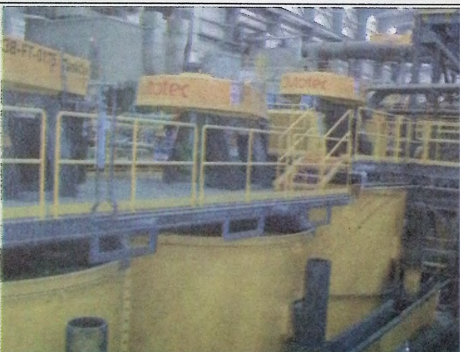
Tank cells in the concentrator building at Copper Mountain Mine are used to separate concentrates. Visitors got an up-close view August 18th at the mine. *
