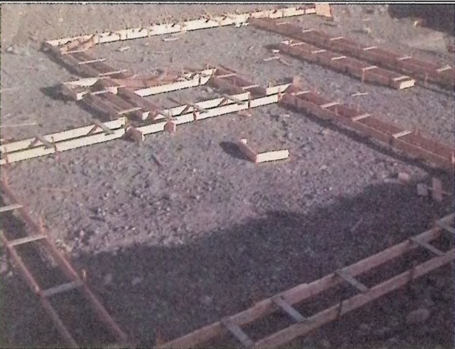
No sooner is one home finished, the 'footprint' of another is laid out at The Yard. This framing will assist builders in laying a concrete foundation. Photo: Brenda Engel
