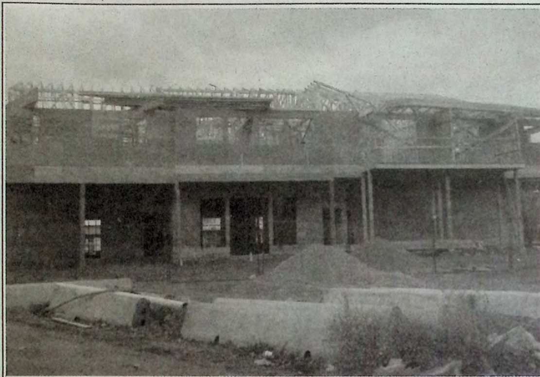
Interest in the Princeton area has led to much new construction in and around town - including this commercial/residential development on Burton Avenue next to Phifer's Fountain. Photo: Brenda Engel
