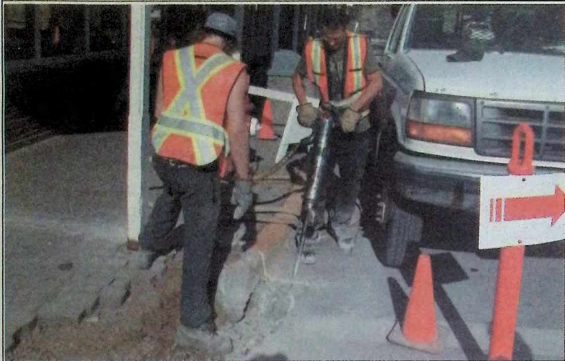
Artistic Imaging Inc. of Revelstoke has the concrete contract for the downtown sidewalk ramps and will be in town at least until mid-October. The company hires locals to assist with all jobs. Photo: Brenda Engel
