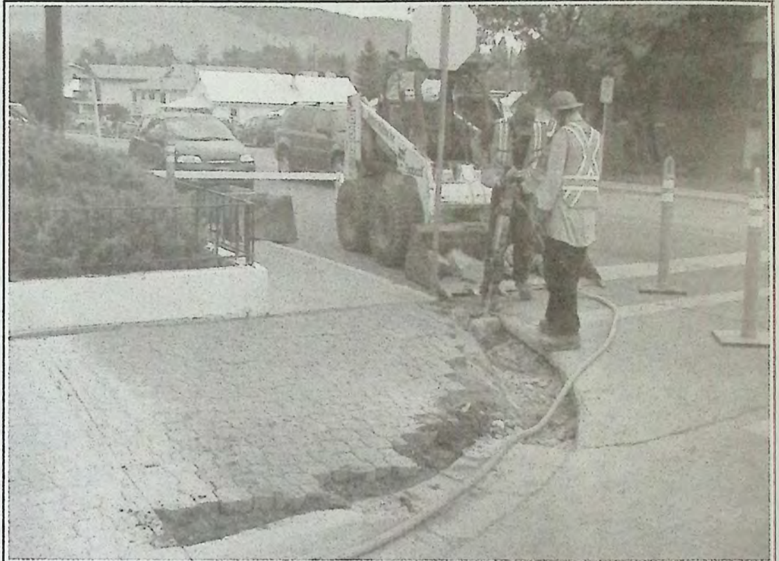
Work continues on upgrading downtown sidewalks with wider ramps. Contractors were busy all last week removing bricks and preparing sites for improvements along Bridge Street. Photo: Brenda Engel
