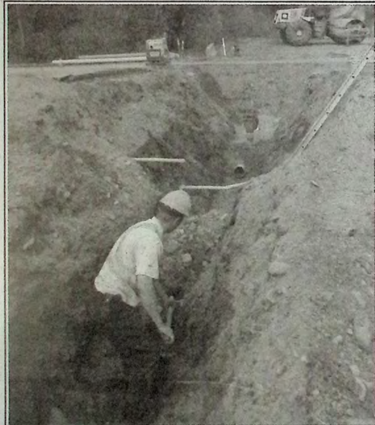
A water line replacement project last week saw crews work across Highway 3 near Billy's Restaurant to the Trans-Canada Trail. Work did not disrupt traffic flow at any time. Photo: Brenda Engel
