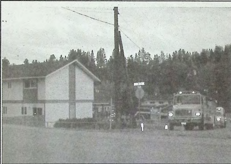
The apartment located at the end of the building (on the left in this photo) suffered extensive smoke damage following a fire at approximately 4:35 PM October 1st in the Aspen Court Apartments at the corner of Tulameen Avenue and Aspen Court in Princeton. No other details were available at press time. Photo: Dawn Johnson
