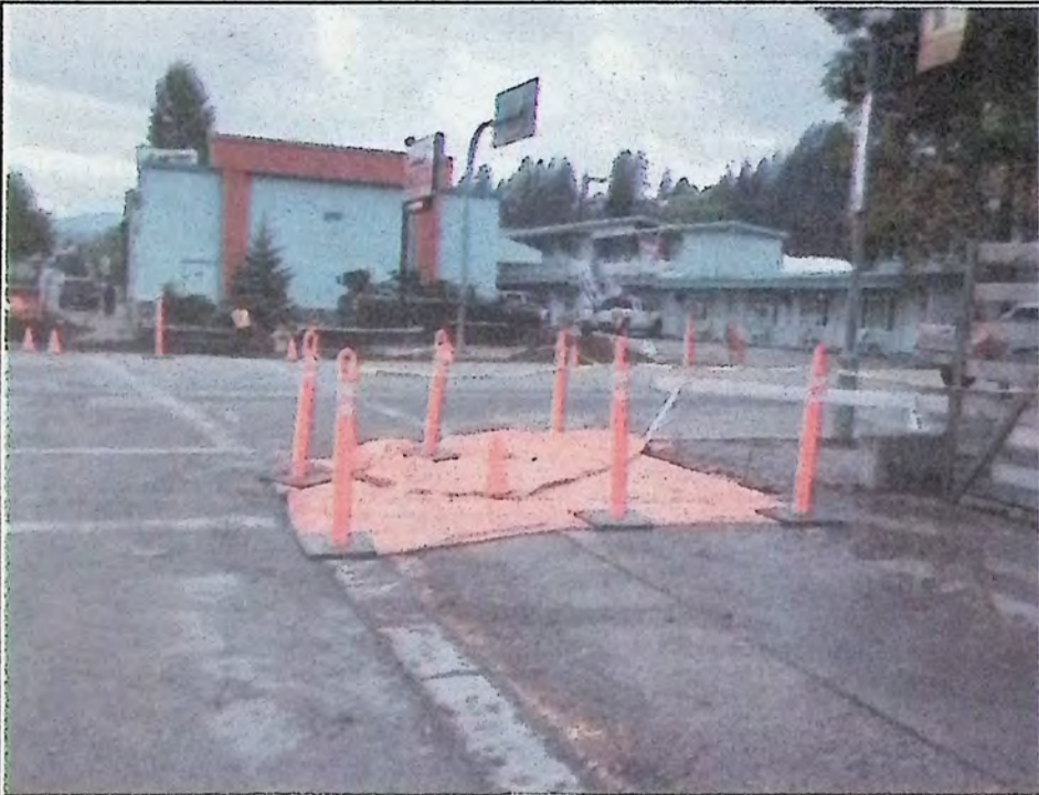
The second phase of the downtown sidewalk ramping project started last week. Two different corners show two different signs of progress on Bridge Street and Tapton Avenue. Photo: Brenda Engel
