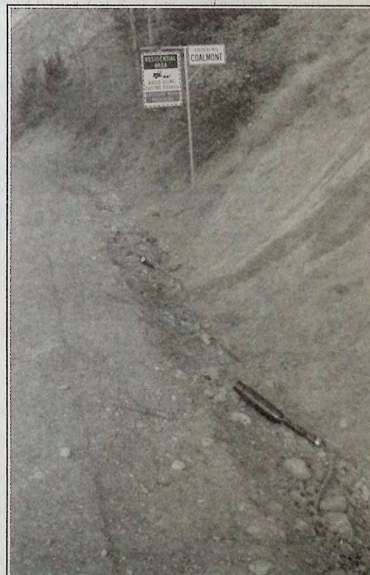
Exposed phone cables along Coalmont Road continue to hamper phone service to the community of Coalmont which does not have access to cell service either. - photo submitted
