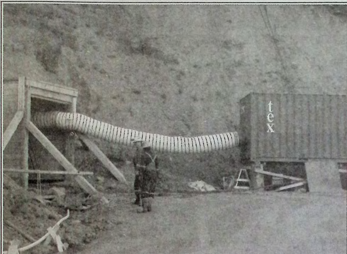
Mine surface infrastructure was installed this year to mine level 1 at Treasure Mountain as part of the ongoing development of the site by Huldra Silver. Photo: Huldra Silver website
