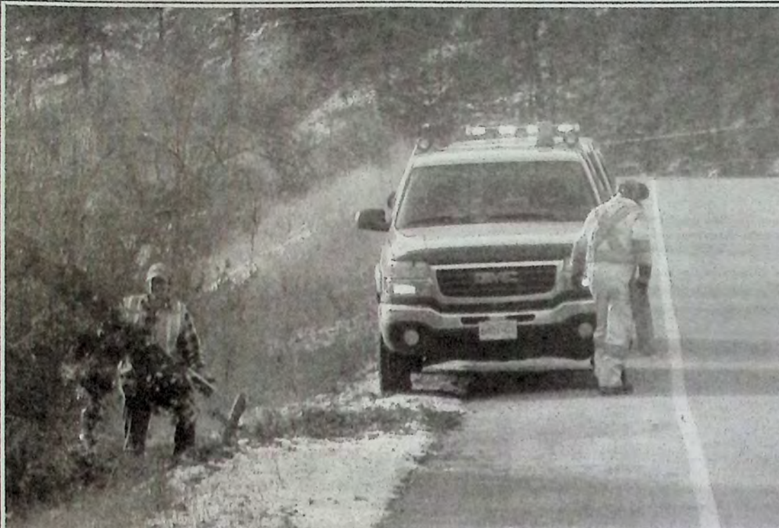
Argo Road Maintenance crew members had the task of sawing and tidying up the trunk and limbs of a giant evergreen on January 12th. The huge tree had fallen across Highway 3A a mile south of the Green Mountain Road, blocking traffic in the wee hours of the morning a few days before. It seems the tree had lived its life on the banks of Keremeos Creek, which - due to the ground moisture content - is inherently soft. When the bulk of the tree was chain-sawed off about five feet from what would have otherwise been its base, the remaining trunk inexplicably popped upright once again! Photo: Arlene Arlow
