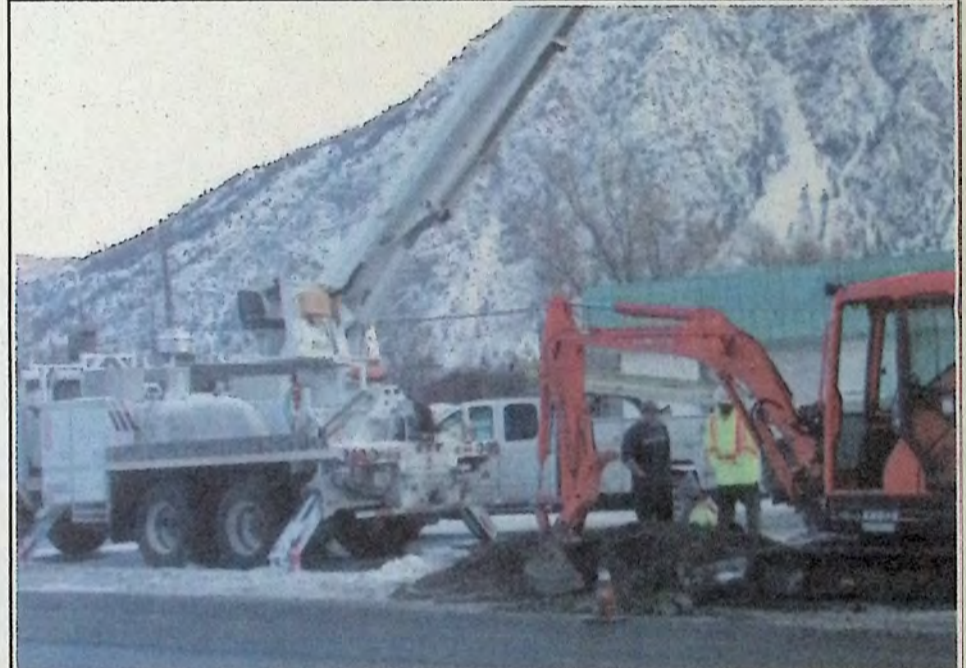
Fortis crews worked January 23rd to stabilize a power pole in Keremeos. The base of the support cable that keeps the power pole from leaning had come loose. The pole had begun leaning sufficiently to compromise the power lines themselves. During the repair, the boom of the Fortis truck was used to prop up the pole. Work was completed without delay. Photo: Arlene Arlow
