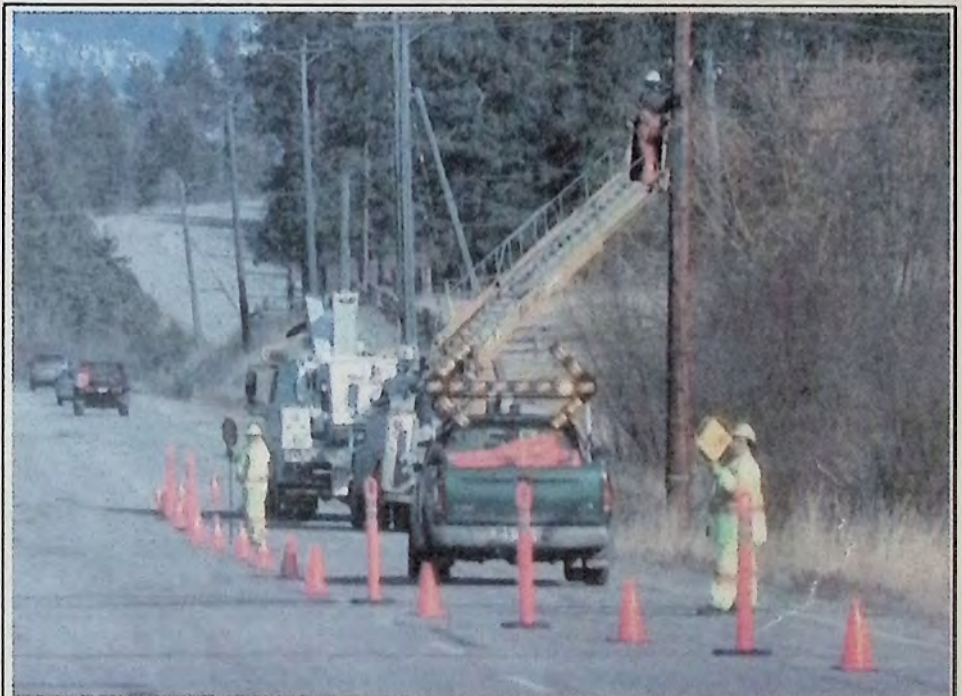
Teamwork! Fortis and Telus crews were busy on Highway 3A February 26th. Looks like a brand-new pole to me. Forget the belt and cleats: a telescoping ladder makes scaling the pole so much easier! Photo: Arlene Arlow
