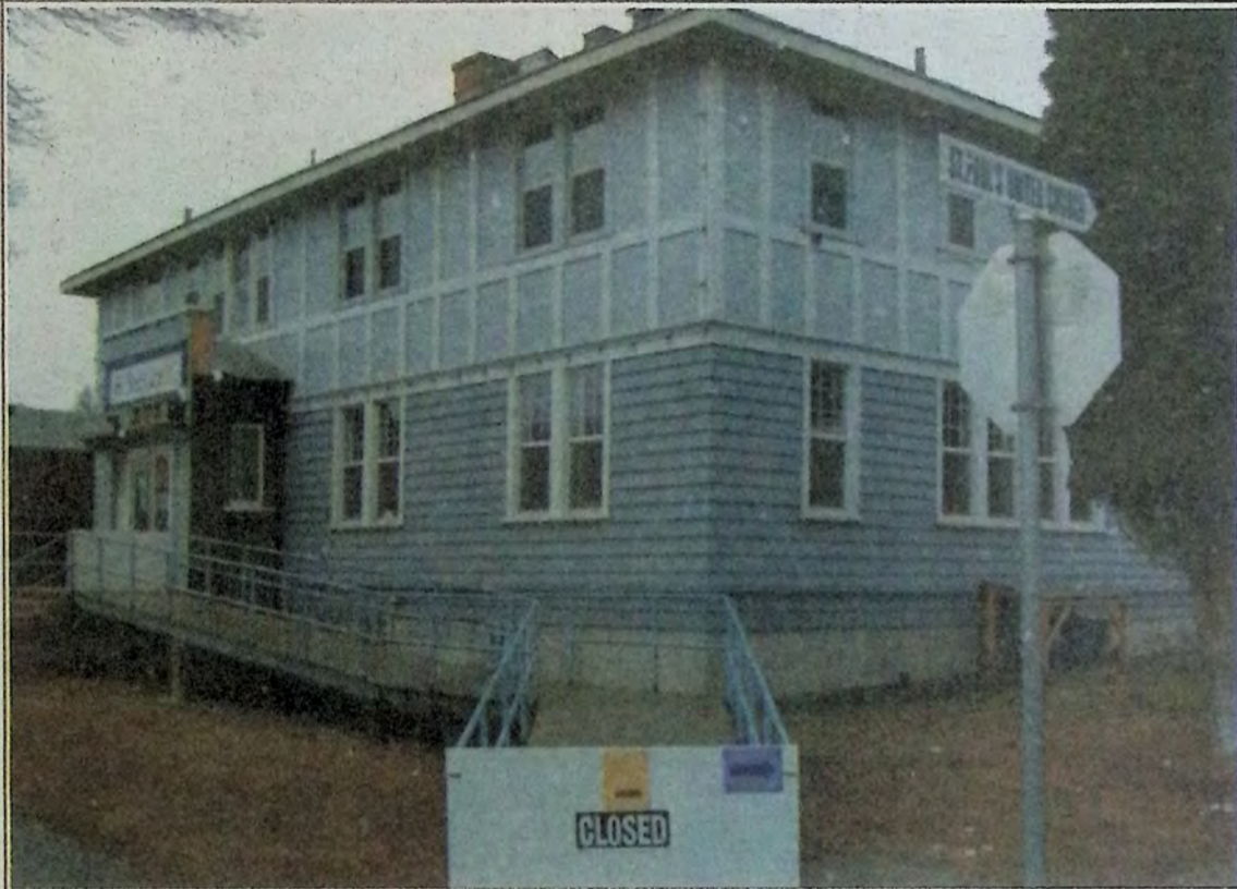
Exterior repairs started March 30th at the Town of Princeton-owned Provincial government service/court house building. While this project has just started, winter doesn't seem to want to end with snow falling daily in the region. *
