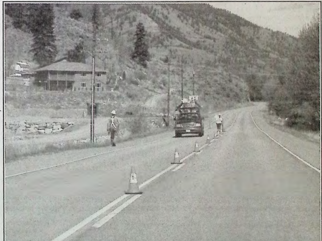
Telus was busy April 24th installing new line to a subdivision just south of Olalla. Safety first: obey all flagpersons. Photo: Arlene Arlow
