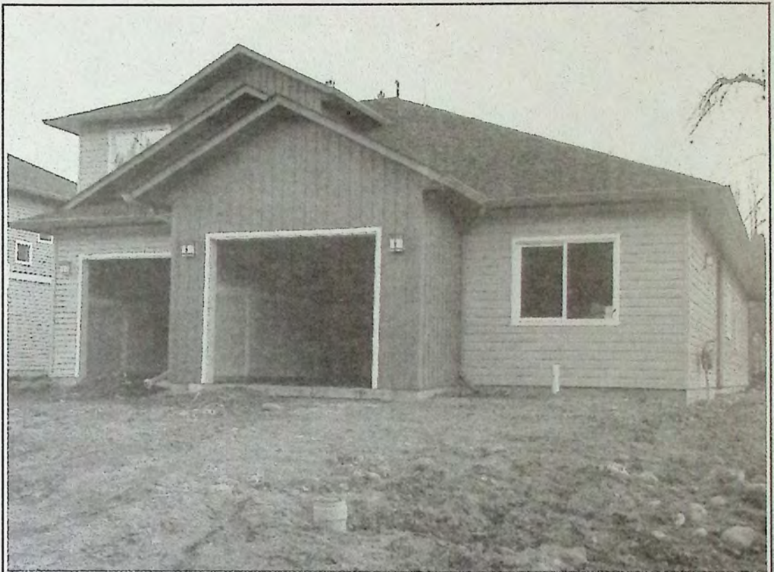
Exactly a month ago this was how construction looked on Similkameen Avenue as part of the Copperstone Homes project. They will host a grand opening celebration this Saturday. Photo: Brenda Engel
