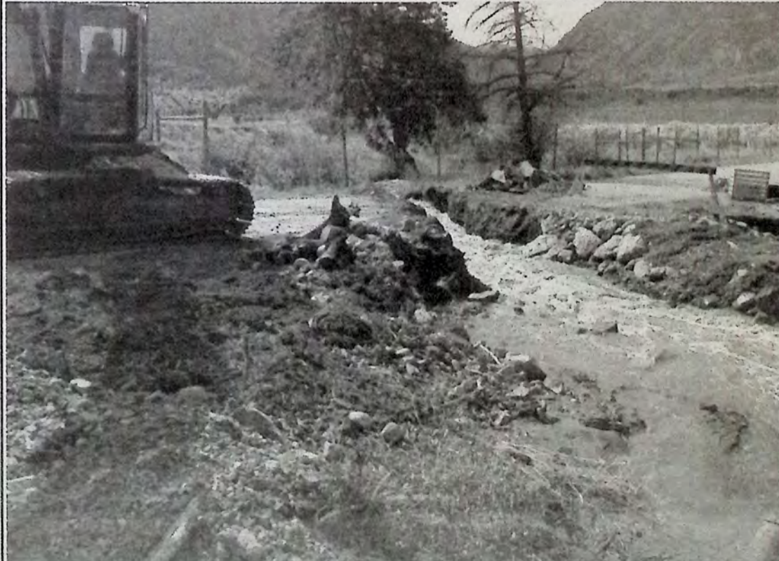
With the warm weather and rains comes flooding. This stream crossing beneath the Upper Bench Road near Keremeos was too much for the culvert. Argo crews cut a new trench parallel to the culvert to minimize damage. Argo Road Maintenance advises that the road is once again open and repairs to that site are ongoing. Photo: Arlene Arlow
