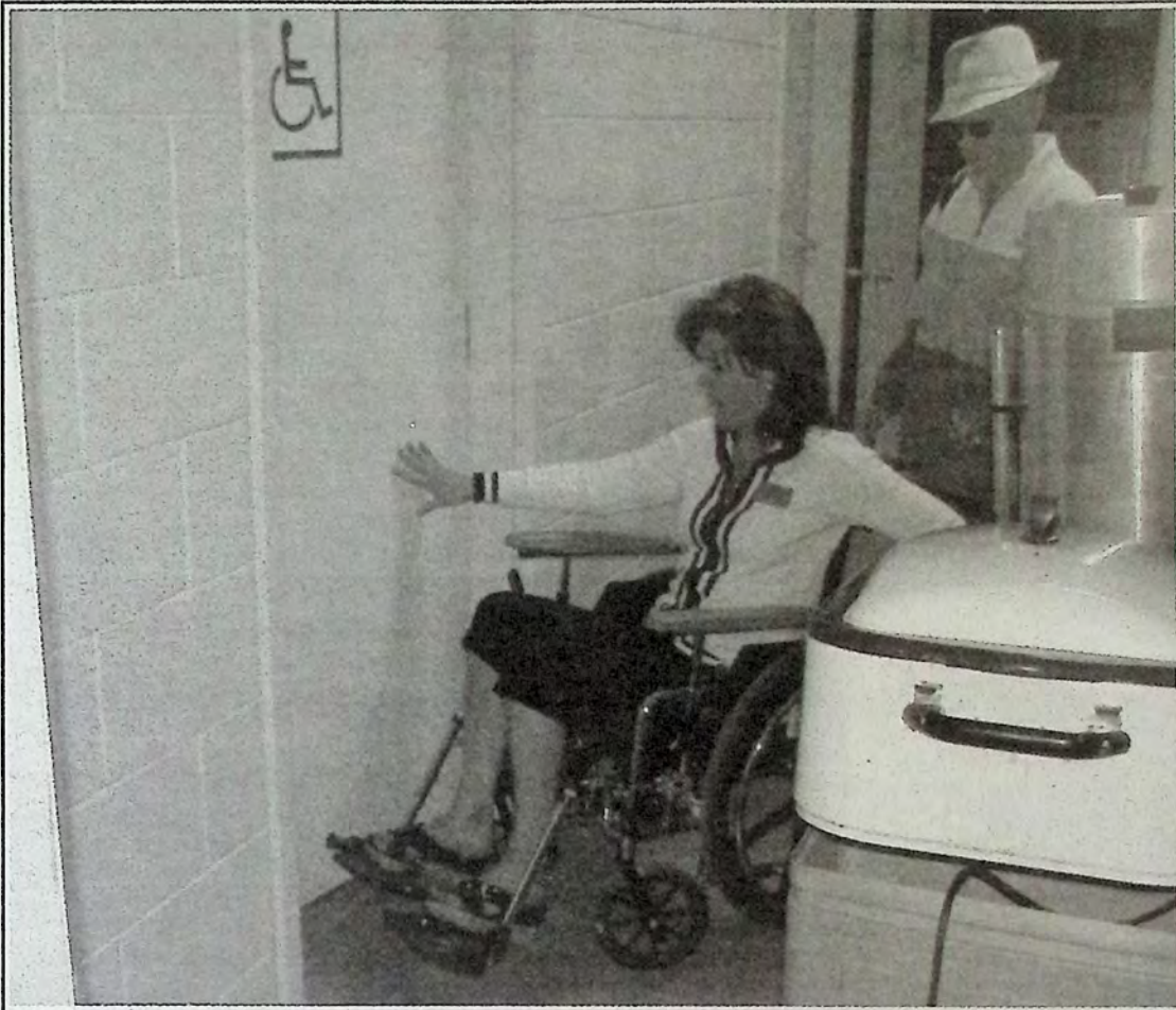
Heather Johnson of Century 21 Princeton Realty, discovers the new washrooms at Princeton Legion Hall are spacious and easy to access from a wheelchair. Johnson, seen here with assistant Mary Bird, was one of a handful of participants in the Princeton Accessibility Awareness Committee's 'wheel about' exercise held on May 9th. *
