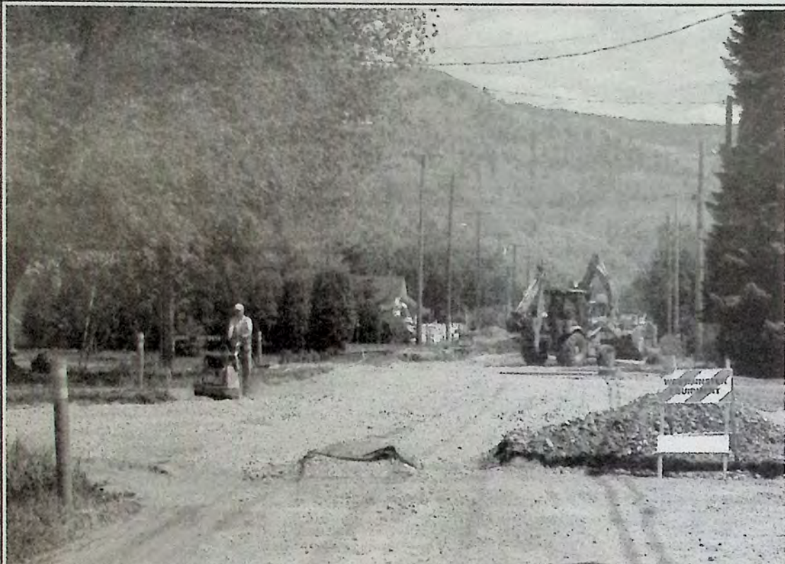
2012 road work has finally begun in Keremeos. Employees from Harris and Son Transport were busy May 18th on 10th Avenue. Other work includes part of 12th Avenue and an alley between 10th and 11th Avenue. Photo: Arlene Arlow
