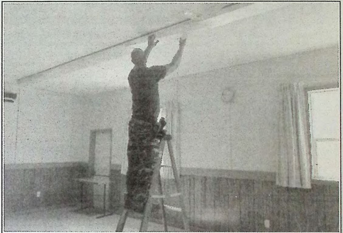
Energy efficient light fixtures were installed May 26th at Cawston Community Hall. - photo submitted
