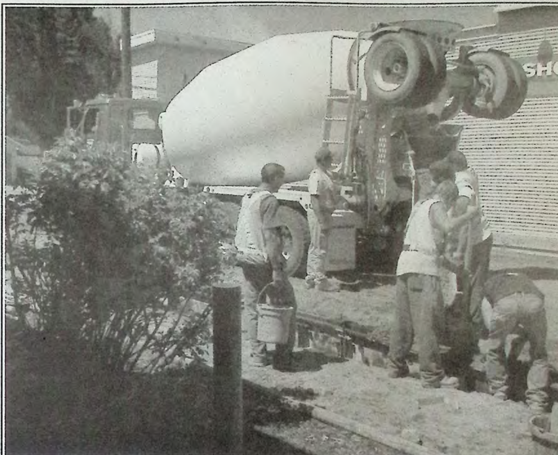
Work on the zig zag project last week included sidewalk curbing. Photo: Brenda Engel
