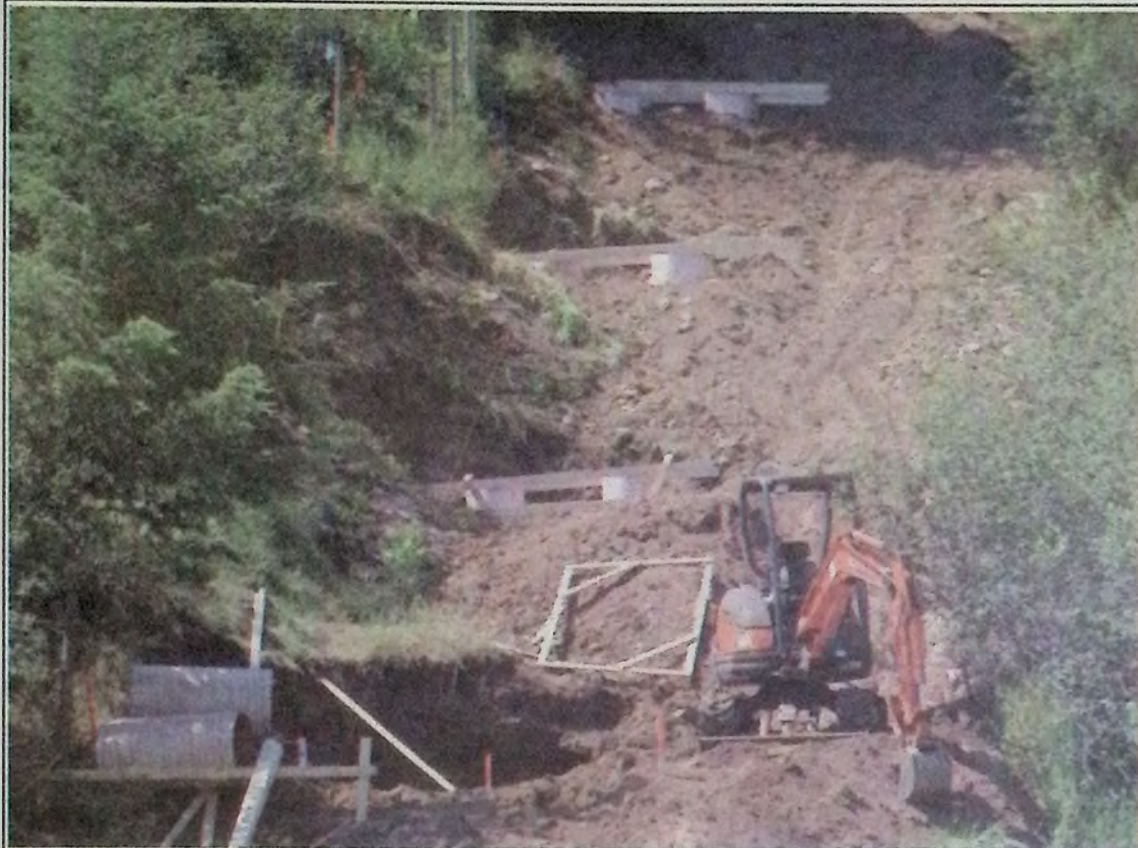
Progress continues on the zig zag project with forms being placed July 6th for concrete pillars. *
