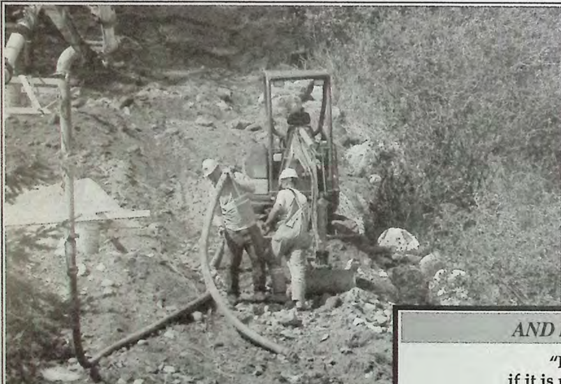
Construction workers used a crane to pour concrete in footings located along the location of the zig zag project July 17th. Photo: Brenda Engel
