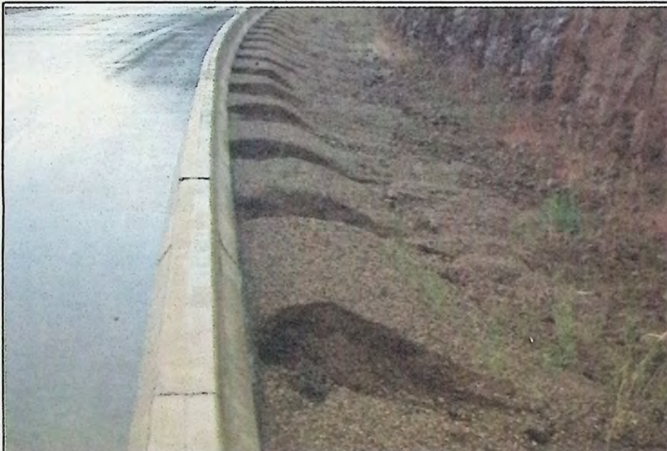
"I wonder if the road edge is supposed to erode like that?" Things you don't see unless you get out of your vehicle: the cement barricades along both sides of Highway 3A at Yellow Lake were manufactured to let water pass underneath at regular intervals. With the unusual downpours that the Similkameen and Okanagan valleys have experienced this summer, the fine rock at the edge of the highway away from traffic has eroded completely up to the edge of the pavement. Photo: Arlene Arlow
