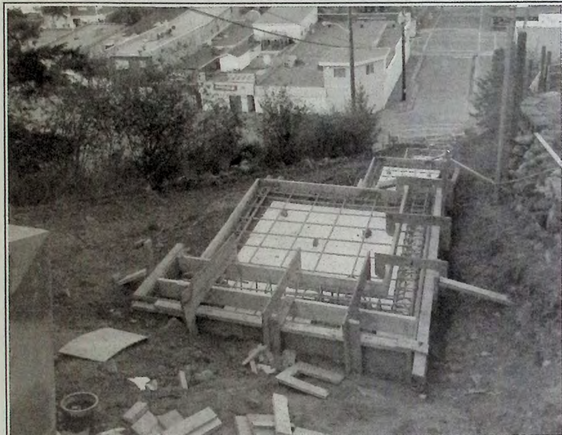
Looking down from the top of the zigzag project the landings are set for cement. This photo, taken the evening of August 16th, gives a better sense of the scale of the project than viewing it from downtown. *
