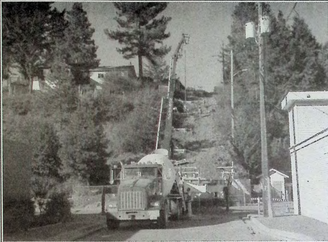
The cement crane was back in Princeton August 17th as crews poured concrete for the landings on the zigzag. *
