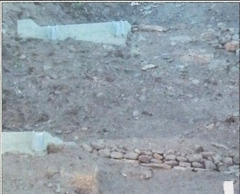
A closer look at some of the rock work being used to shape a trail between landings. *
