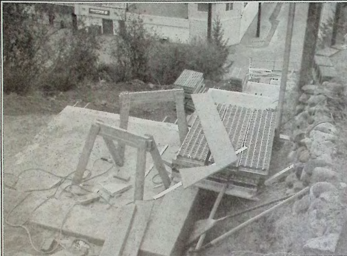
Looking down from the top of the zigzag September 5th. Note the piles of steel treads stacked ready for installation. *
