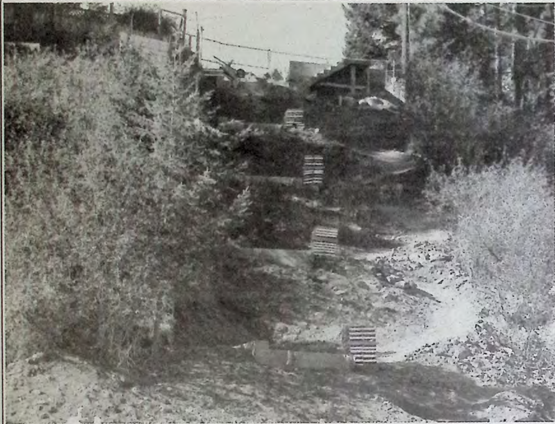
Progress continues to show daily on the zigzag project. On September 11th it was easy to see the 'zigzag' path which runs to the right of the stairway down the slope between First Bench and downtown Princeton. *
