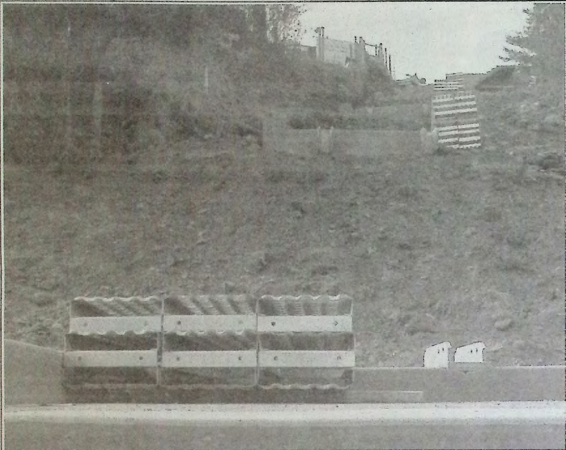
There was no further work done last week on the zigzag project from First Bench to downtown. In the foreground is the bottom landing of the new project with stair treads stacked ready for installation. *
